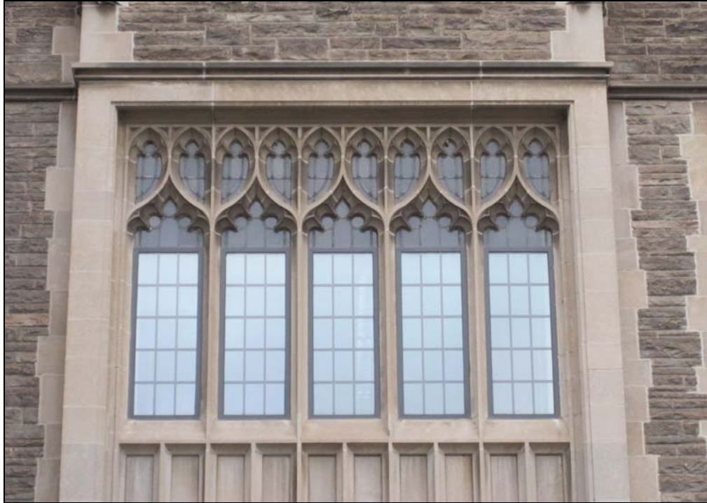
Hamilton Hall - windows replaced in 2002 with aluminum windows similar to those currently proposed for University Hall.
