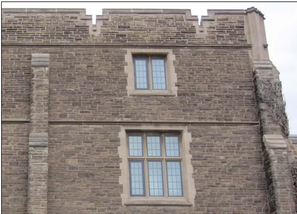
Hamilton Hall - lower sashes replaced in 2002, note the mix of operational, casement window and fixed windows
