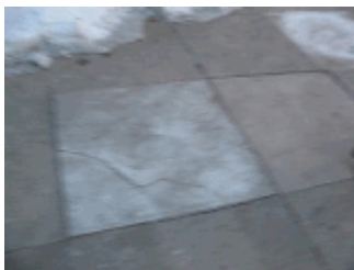
Deteriorated sections where attempts to restore have been undertaken.
