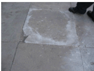
Unrepaired deteriorated units observed during the assessment on the Queenston walkway.
