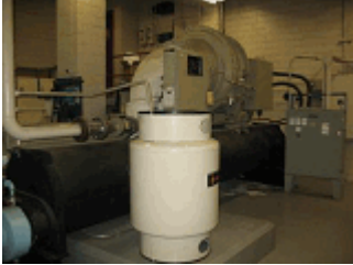
Centrifugal chiller installed in 1990.
