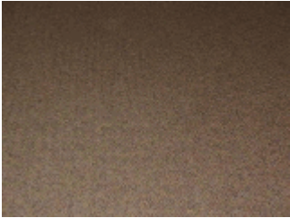
General condition of the carpet observed during the assessment.
