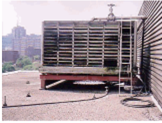
View of cooling tower on main roof
