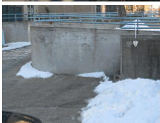
Hairline cracks on the planter boxes retaining wall adjacent to the concrete ramp.
