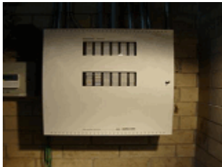
Main fire alarm control panel
