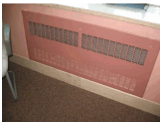
Typical forced flow heaters provided in the some offices.
