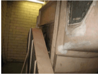
Return fan in the mechanical penthouse.
