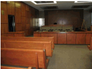
Condition of the carpet in the Ontario Municipal Board room located on the 1st floor not replaced in 2007.
