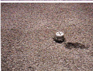
View of roof drain on BUR requires replacement.
