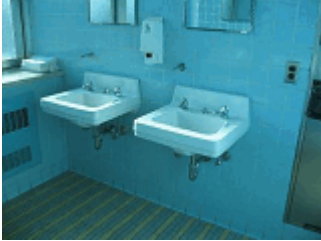
Typical ceramic sinks in the washrooms. The faucets dispense separate hot and cold water.
