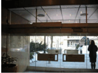
Front Entrance Doors. The exterior doors are glass doors with pivot hinges.
