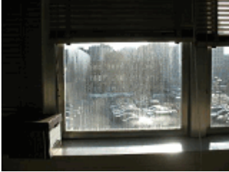
Failed IGUs observed during the assessment.
