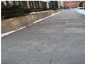
General view of the Queenston walkway provided to the north of the building.
