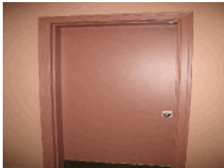
Typical hollow metal doors. The doors were restored to remediate suspect hazardous containing materials.
