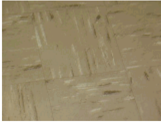
Vinyl floor tiles provided in the building.
