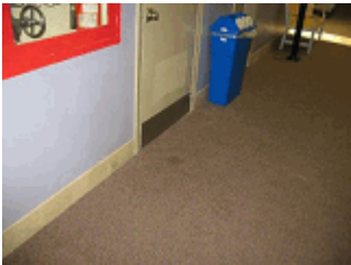
Some staining as result of usage observed on the carpet.
