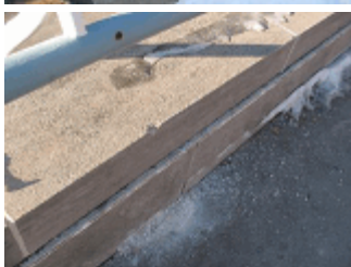
Closer view of the displaced stone cap on east property perimeter.
