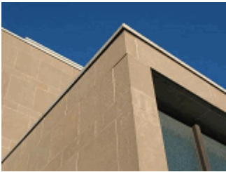
Movement of the stone facing observed on the south elevation.
