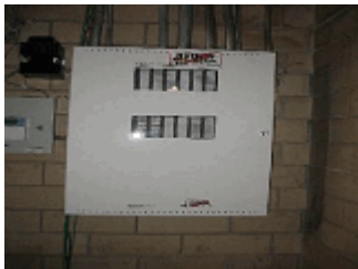
Fire alarm manufactured by MirCom. Unit installed in 2004.
