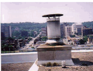
View of boiler stack
