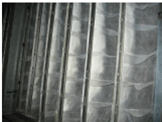
Bag filters that replaced the abandoned precipitron.
