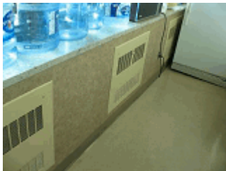
Perimeter forced flow heaters provided in the kitchenettes on each floor.
