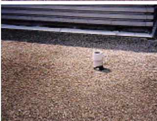
View of Flashing at Cooling Tower will require replacement when BUR is replaced.
