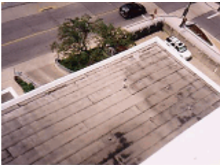
Lower modified bitumen roofs have evidence of ponding and seams are in poor condition.
