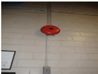
Fire alarm bells located throughout building
