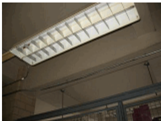
Original light fixtures with T8 lamps
