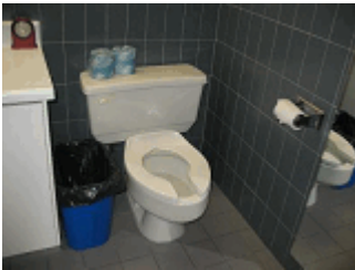
Typical toilet bowl with flush tank.
