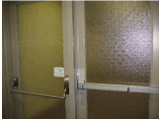
Glass doors in aluminum frames.
