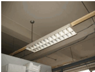
Original light fixtures with T8 lamps.
