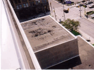
View of lower modified roofs, poor condition, requires replacement.
