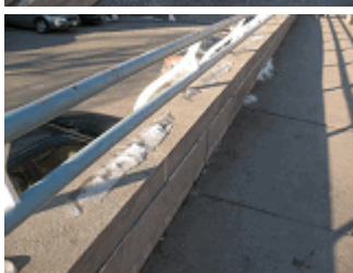
Displaced stone cap on east property perimeter.
