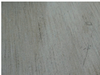
Closer view of the sheet vinyl floor covering provided in the kitchenette.
