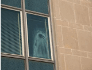
Failed IGUs. Moisture infiltration has occurred.
