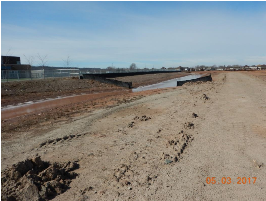
Photo 3 – looking west - large ditch behind elementary school
