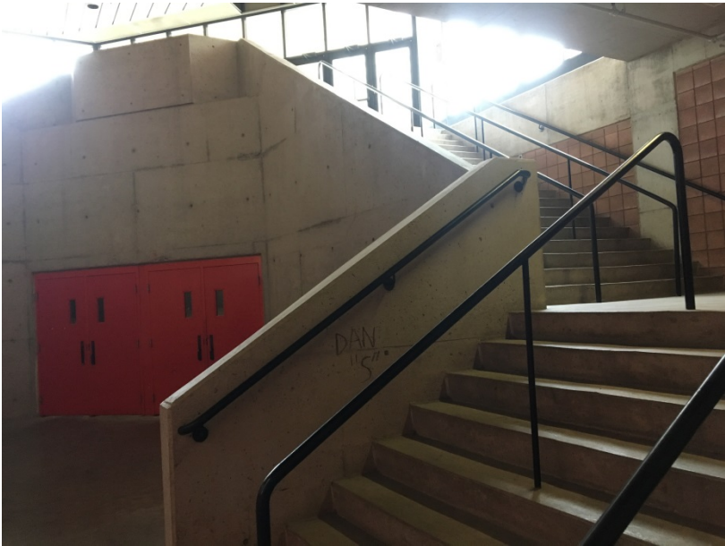
Doors Accessing to Escalator #5 from Escalators #6 & #7
