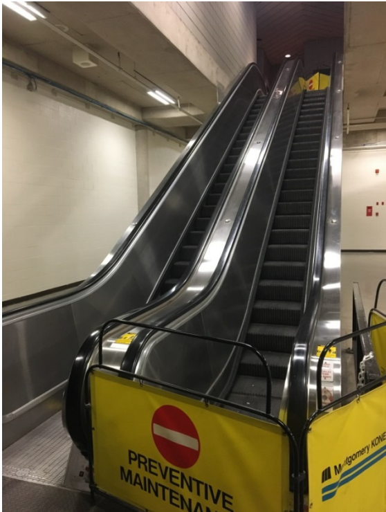
Escalators #1 & #2 Lower/Rink Level to Ground Level
