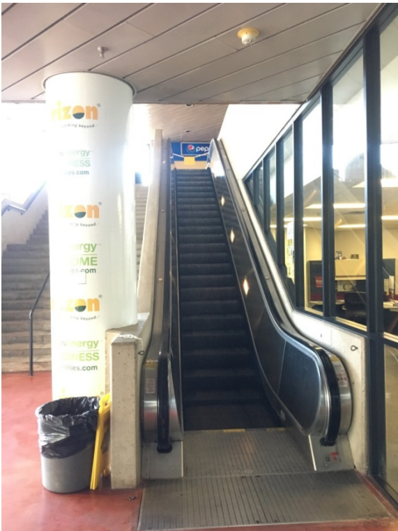
Escalator #3 – Bay Street North
