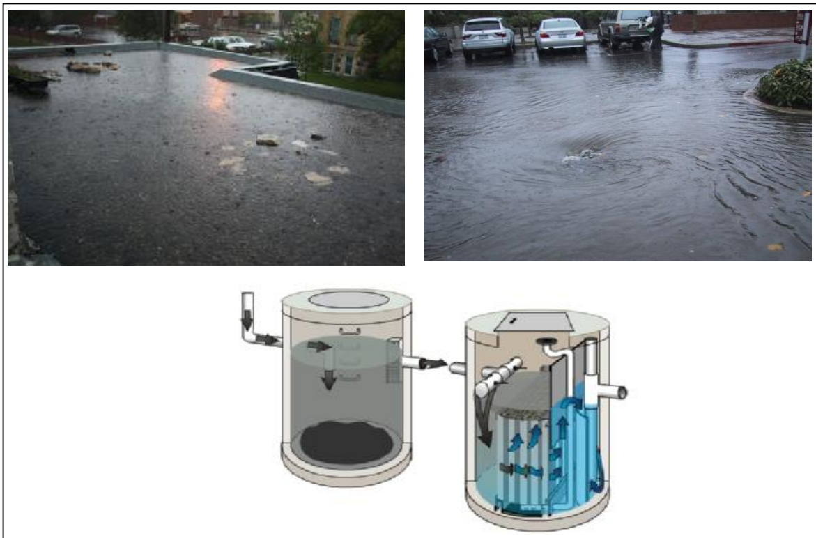
Figure 6.1: Traditional Source Controls (Clockwise, from top left: Rooftop Storage, Parking Lot Storage, Oil-Grit Separator)
