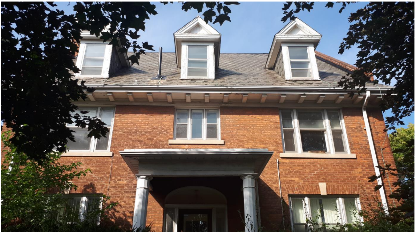
Figure 2: A closer view of the symmetrical southern façade showing the columned portico, window keystones, slate roof, and Classical pedimented dormers (2017).
