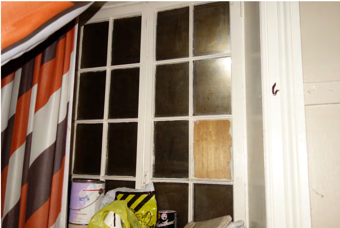
Furnace room window – enclosed under the front stoop
