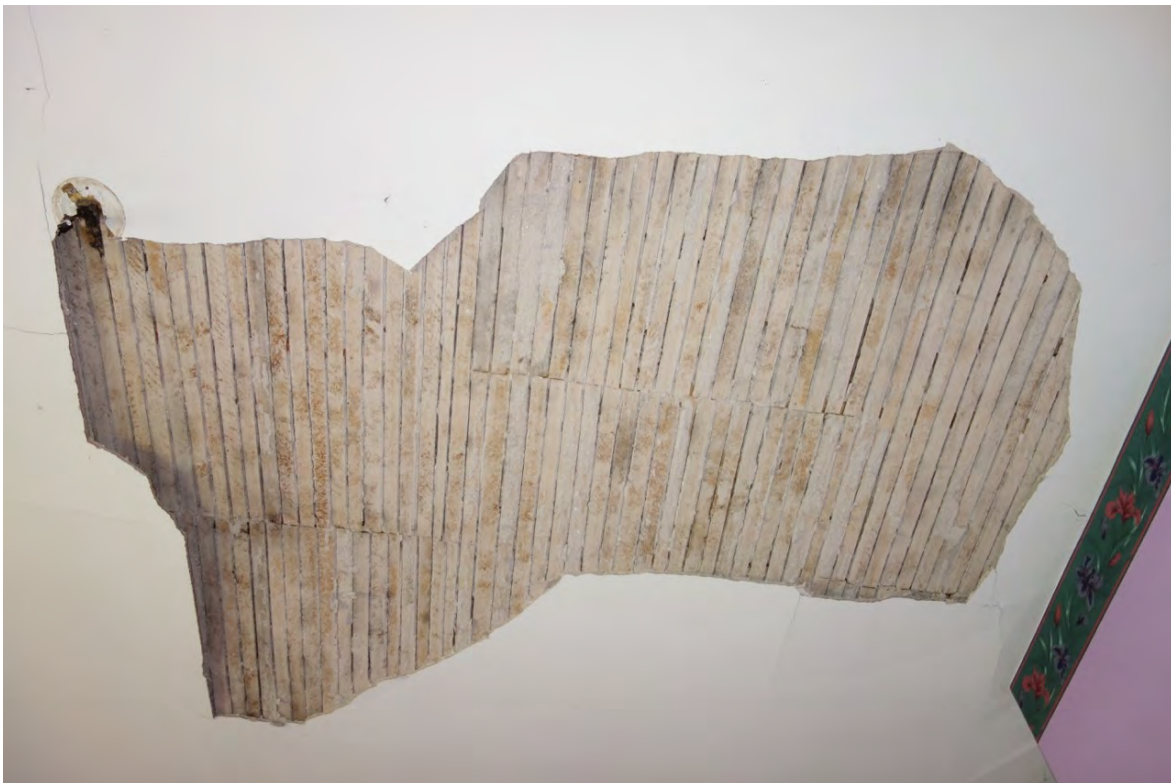
West parlour – ceiling plaster damage
