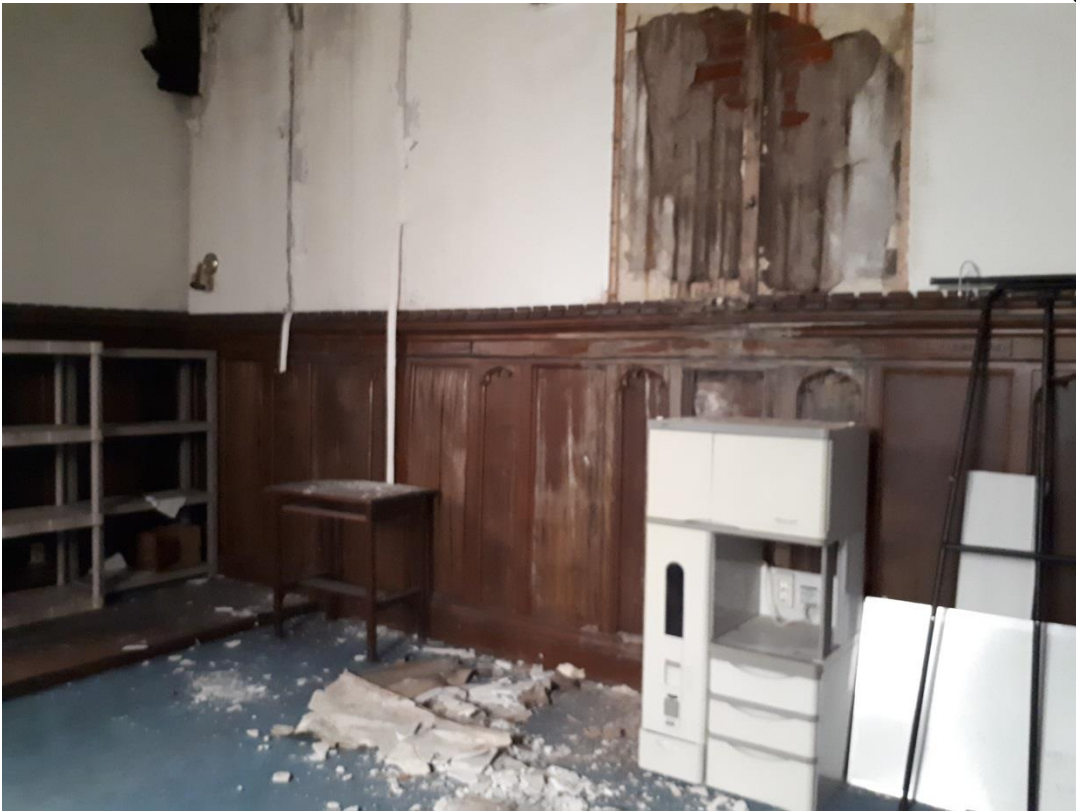
Water damage in Memorial addition, May 31, 2018
