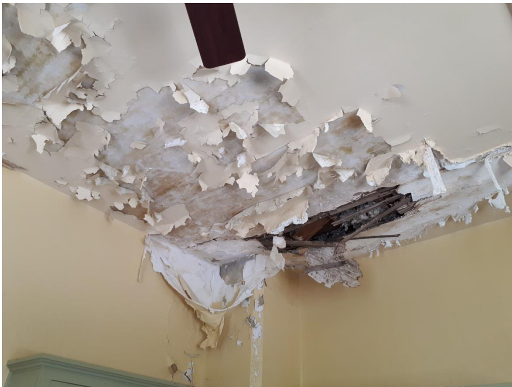
Water damage in room above arched entrance on Holton Avenue South, May 31, 2018
