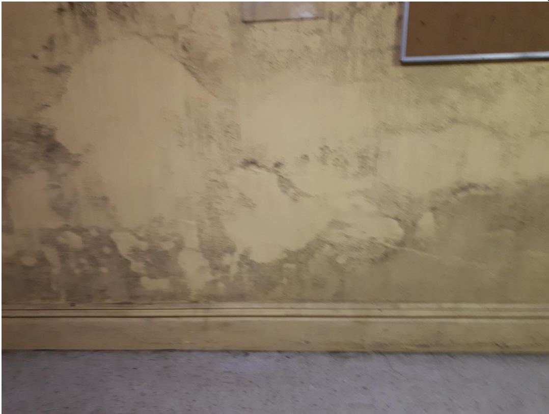
Basement near kitchen, May 31, 2018 (black is mold growth)
