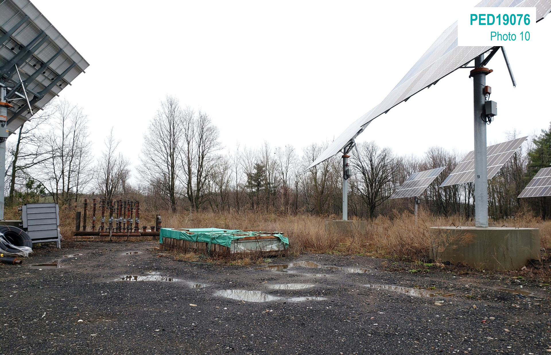
Solar Panels to the south
