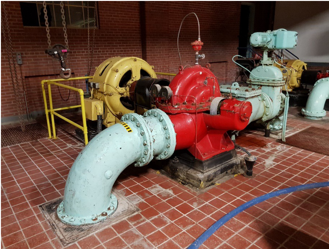
Figure 66: One of five Middle Level Pump Trains in the 1929-30 Extension.
