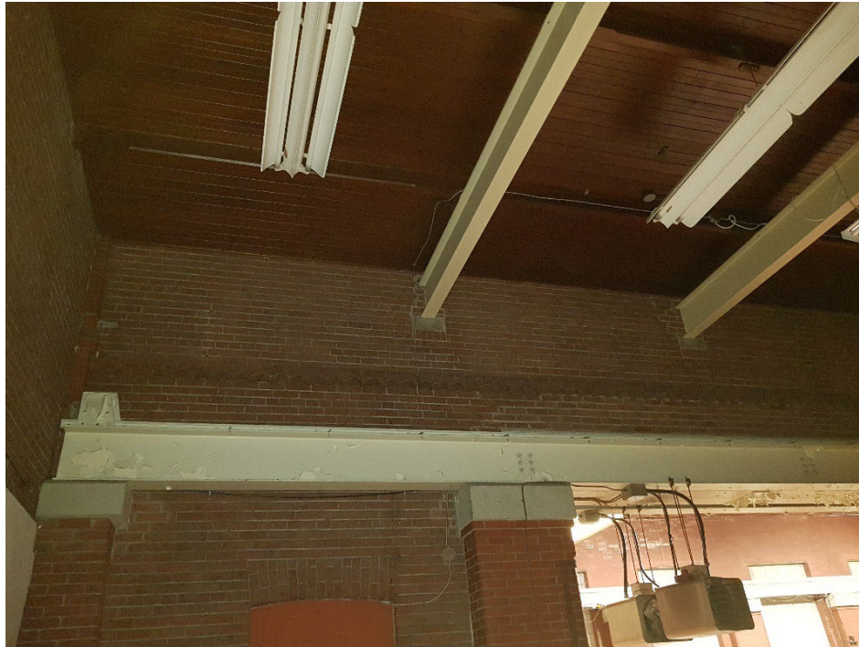
Figure 55: Exterior wall with coggling of the 1912-13 Block as seen from within the 1929-30 Extension.
