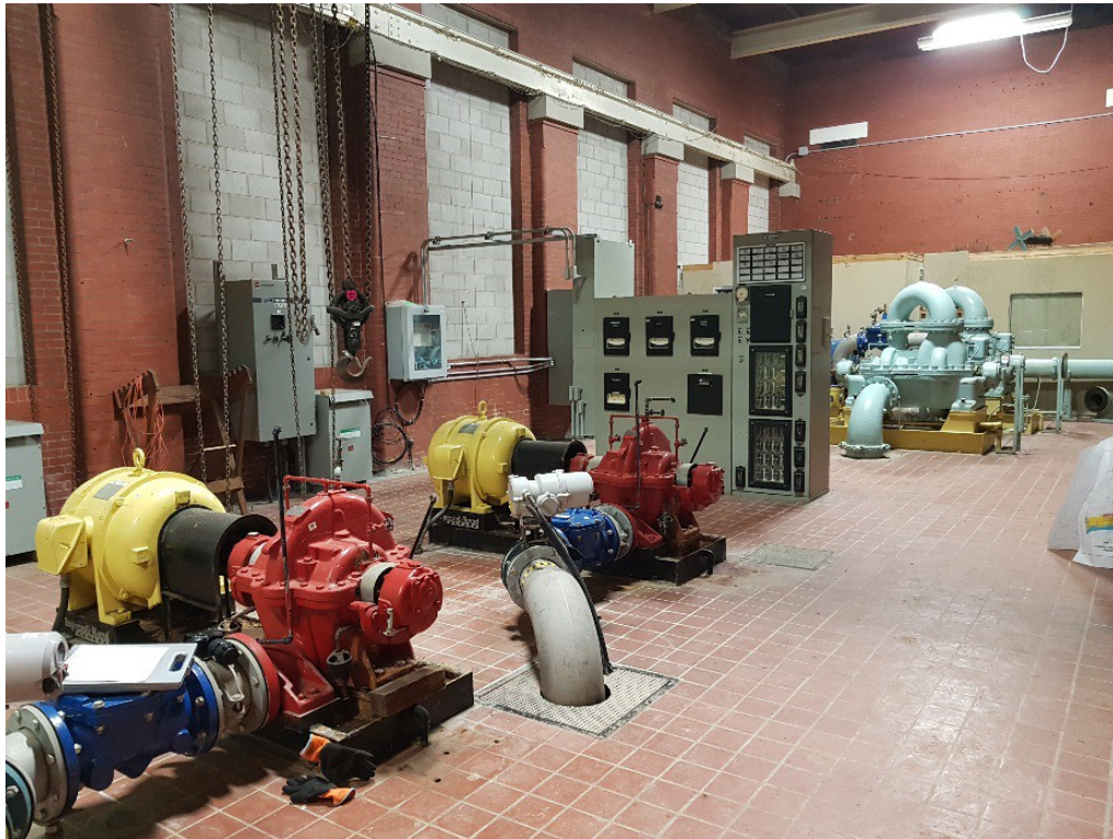
Figure 52: Mountain Level Pump Trains, High Lift Pump Trains, and Control Panel on the north portion of the floor.
