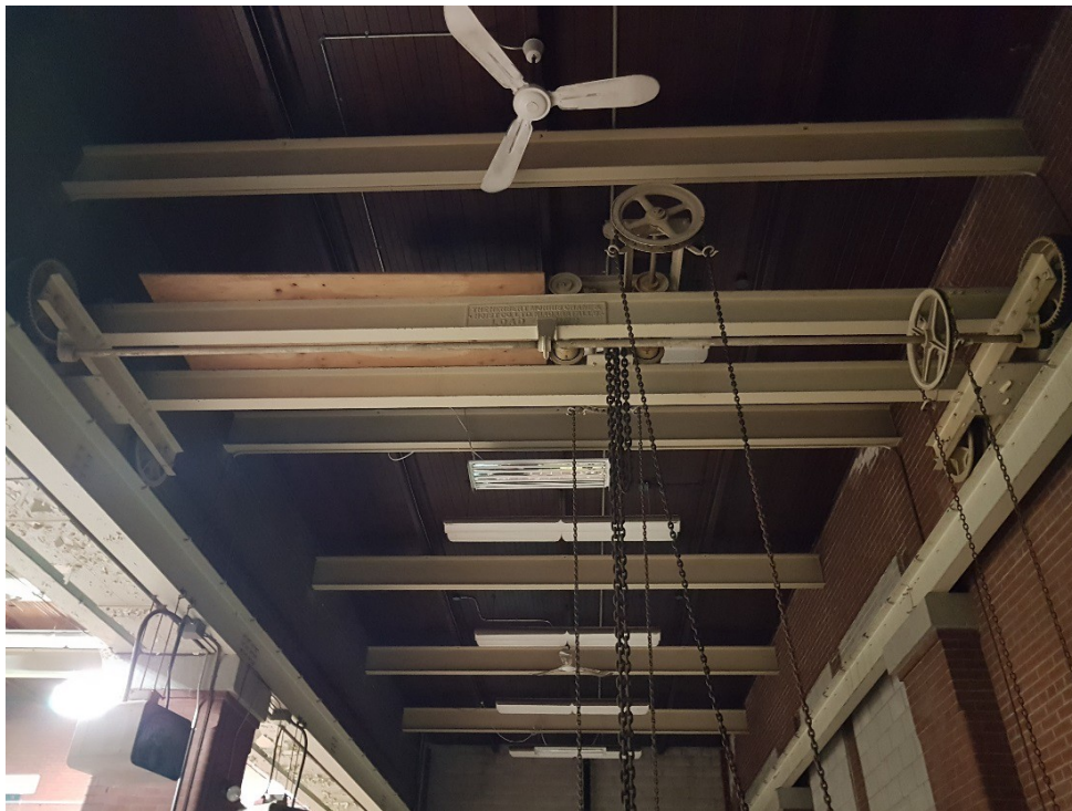
Figure 65: Chain pulley hoists suspended from lateral I-beams with Herbert Morris Chain and Hoist Company Ltd plaque.
