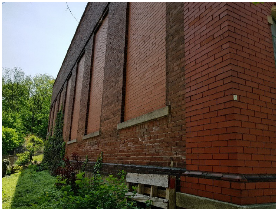
Figure 45: Blind windows and lower quality brick laid in common bond on the north façade. Note also the cogging course above the windows.
