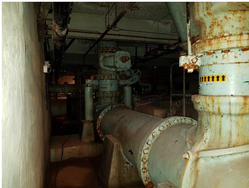
Figure 67: View facing east of the piping beneath the 1929-30 Extension.
