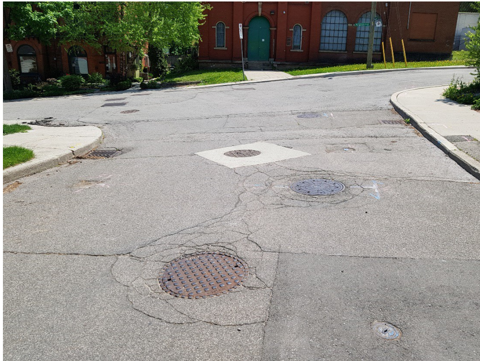
Figure 30: Numerous round and square maintenance covers west of the Ferguson Avenue Pumping Station.
