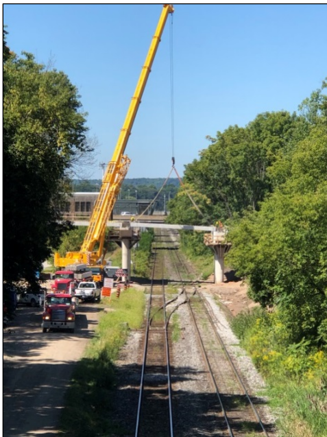
Widening the John Street bridge allows us to expand GO Train service to Hamilton
