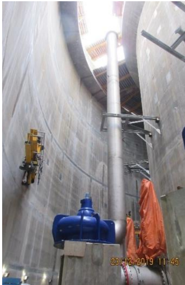
Figure 3: New Pump and Piping
