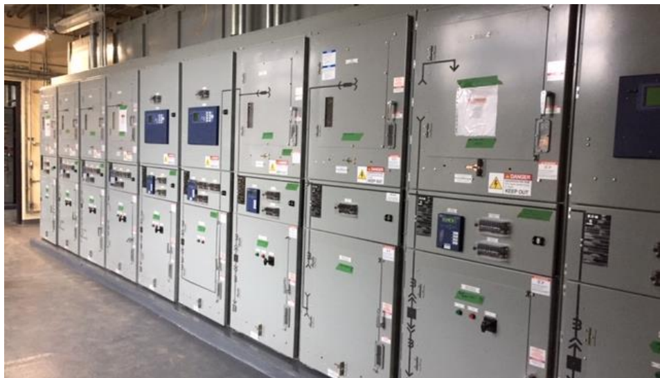
Figure 6: New Switchgear in Electrical Power Centre
