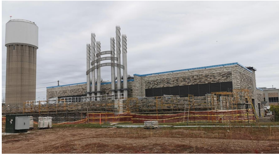
Figure 4: New Electrical Power Centre
