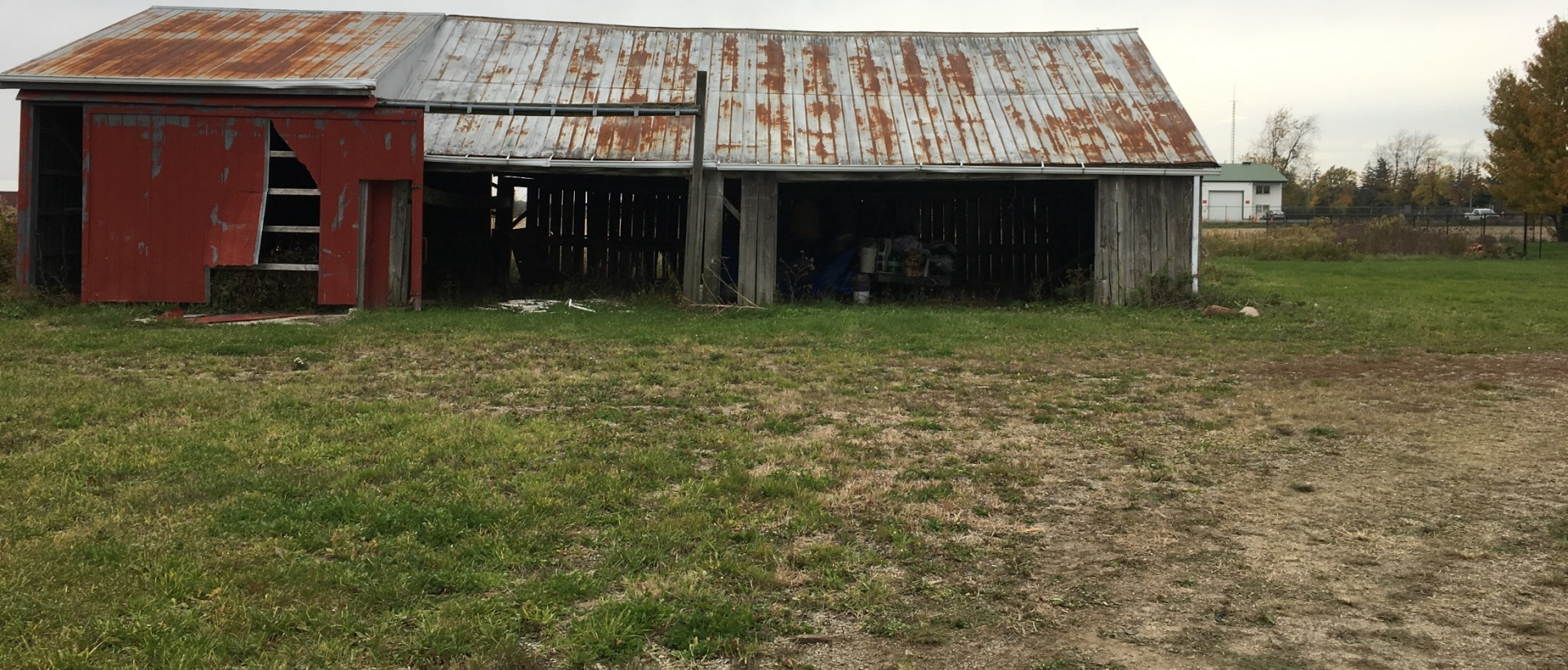
One of the barns that will be demolished as part of the approved severance application
