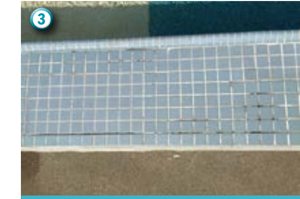
3 Wave pool surfacing and tile is degrading, potentially leading to sharp debris in the wave pool, posing a safety risk.
