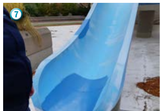
7 The slides and pool surfacing in Squirt Works is visibly degrading.
