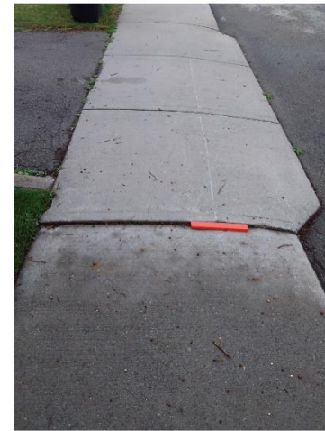
Trip Hazard Deflection
