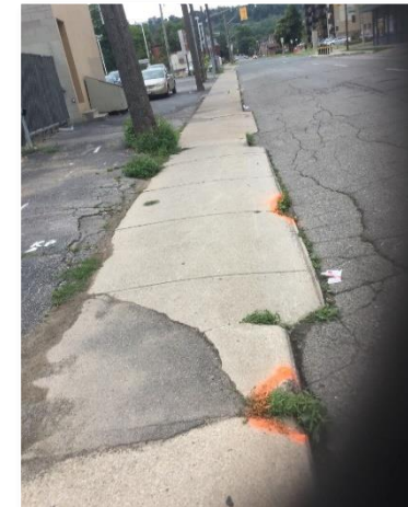
Uneven Surface Deflection 75
