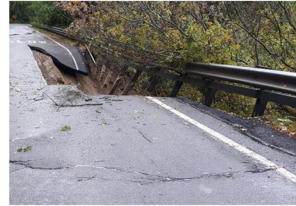
Hwy 8 Dundas Escarpment Failure
