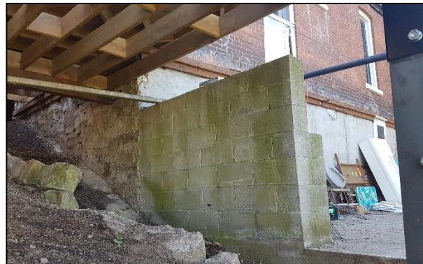
Figure 23: Wooden deck, concrete block wall and poured concrete behind the residence (ASI 2020)
