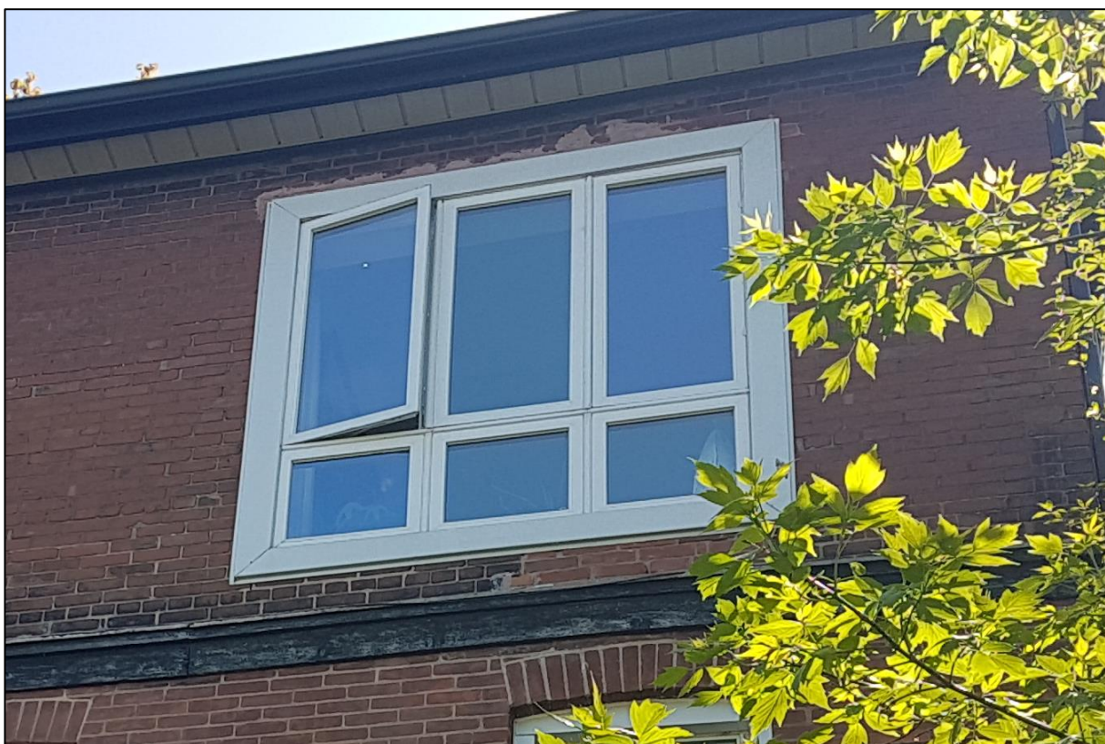
Figure 21: Detail of the enlarged second storey window on the rear elevation (ASI 2020)
