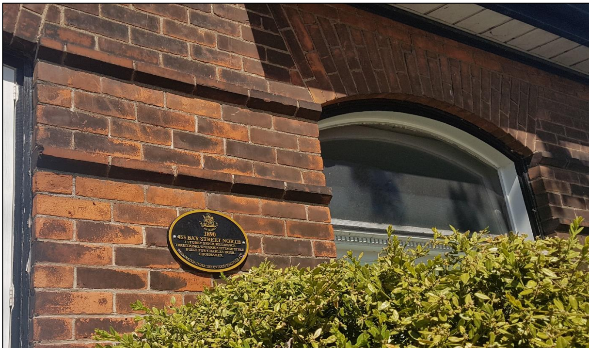
Figure 15: Detail of the building's plaque, brick banding and flat arch above the window (ASI 2020)
