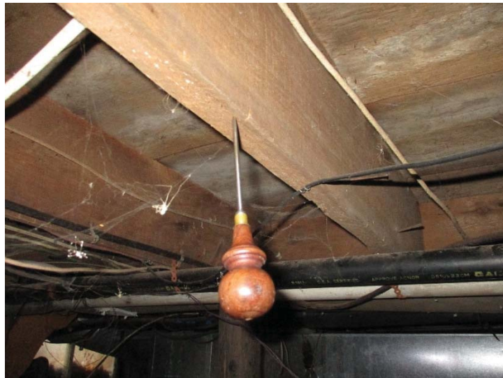
Deteriorated floor joist, awl inserted >2"
