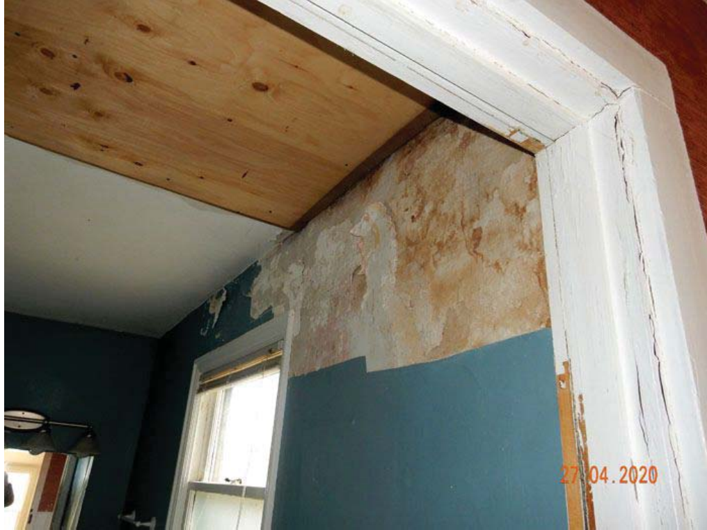
Figure 10: Interior Ground Floor New Trim and Damage Ceiling and Plaster, 1389 Progreston Road
