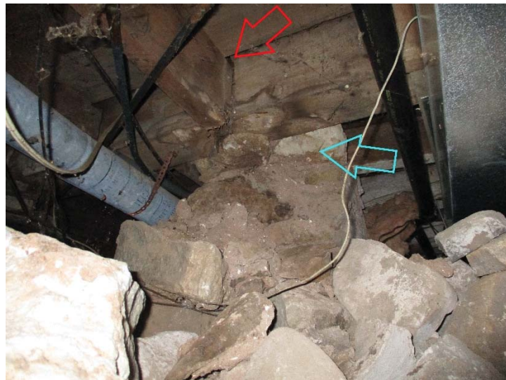
Dropped joist, sawn timber sill plate, altered foundation, missing support
