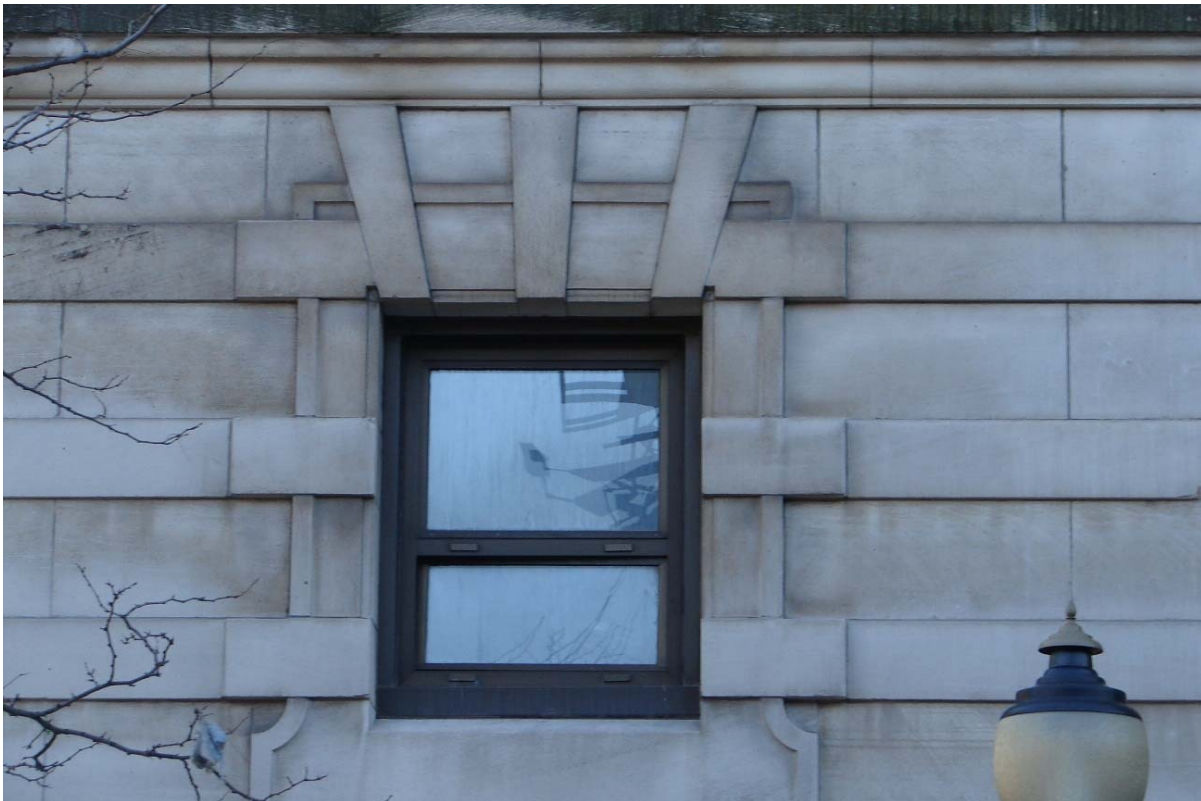
Fig. 45 Mezzanine-floor window with quoins and exaggerated voussoirs and keystone for its stone surrounds
