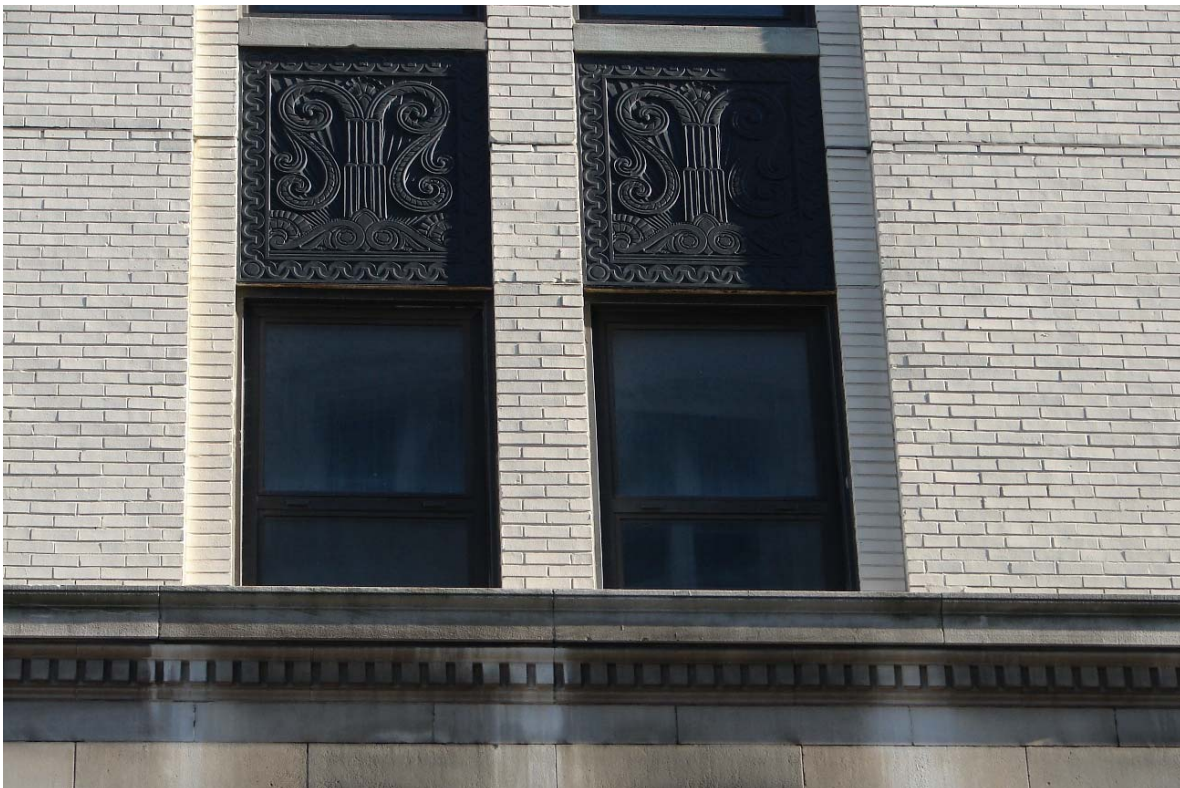
Fig. 75 Windows in west elevation's tower shaft (note bronze spandrels in the Art Deco style)
