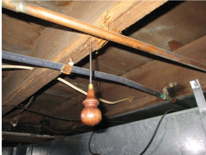
Deteriorated floor joist, awl inserted >2"
