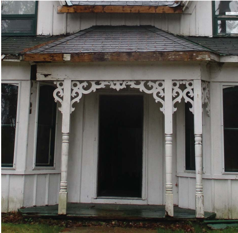
Porch with upside-down posts
