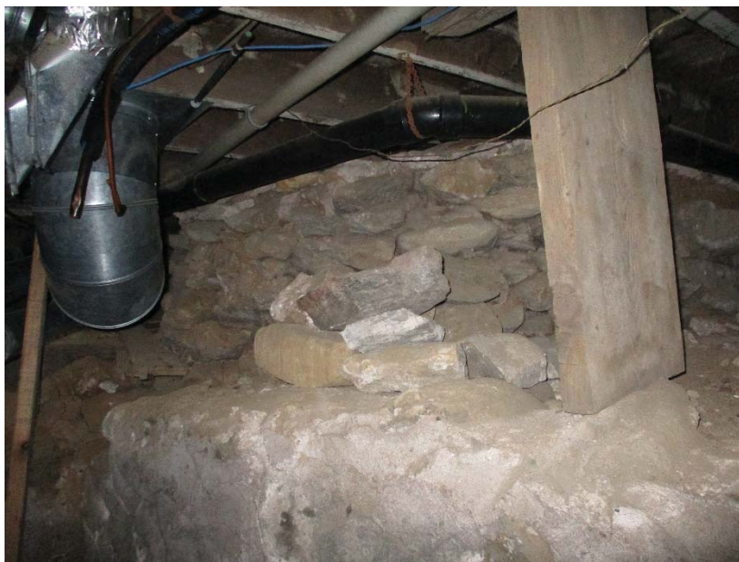
Later basement wall (foreground) supporting earlier shallow wall (background) Also note temporary prop under failing joist
