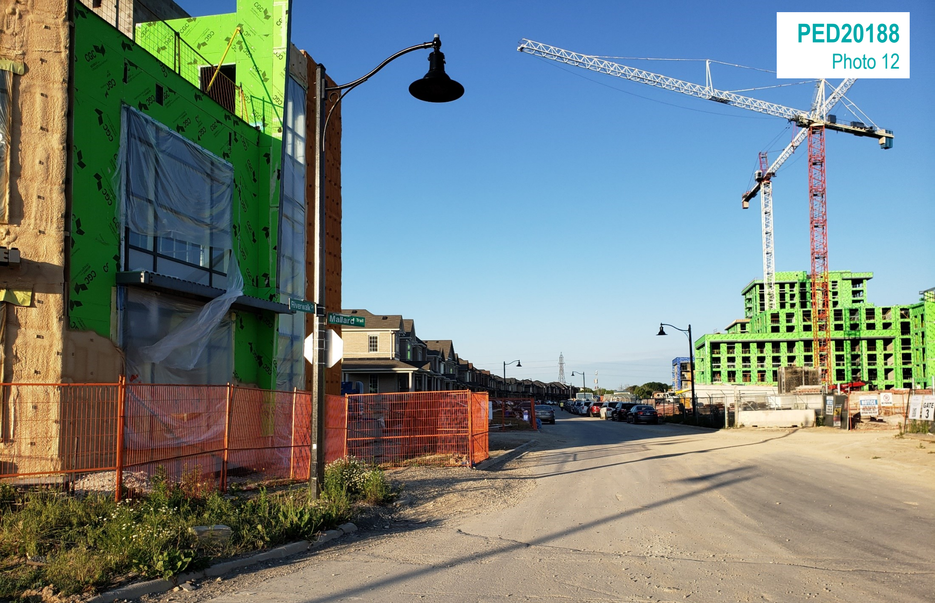
Existing and Proposed Townhouses and Multiple Dwelling to the South
