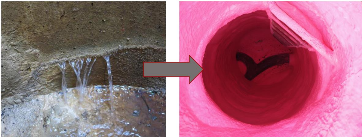
Figure 1.2: Infiltration in Manhole (left) and SpectraShield® Sealant in Manhole to Mitigate Infiltration (Right)
