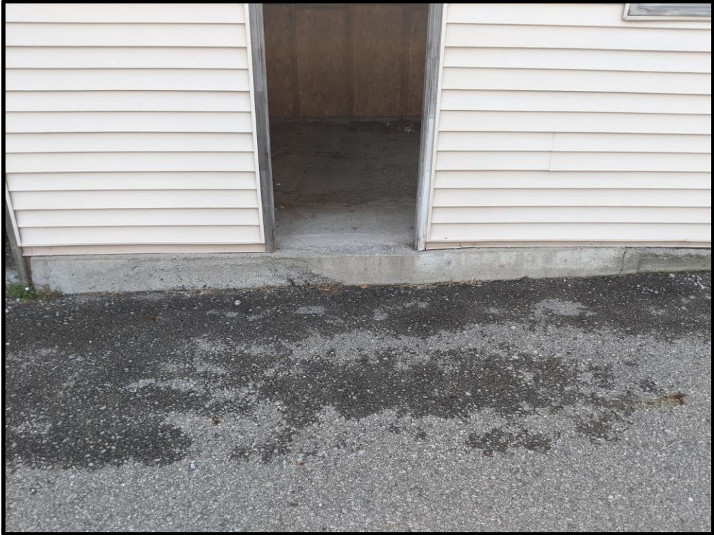
Exterior of Garage and Concrete Pad, 19 Mill Street South, Waterdown City of Hamilton 2021
