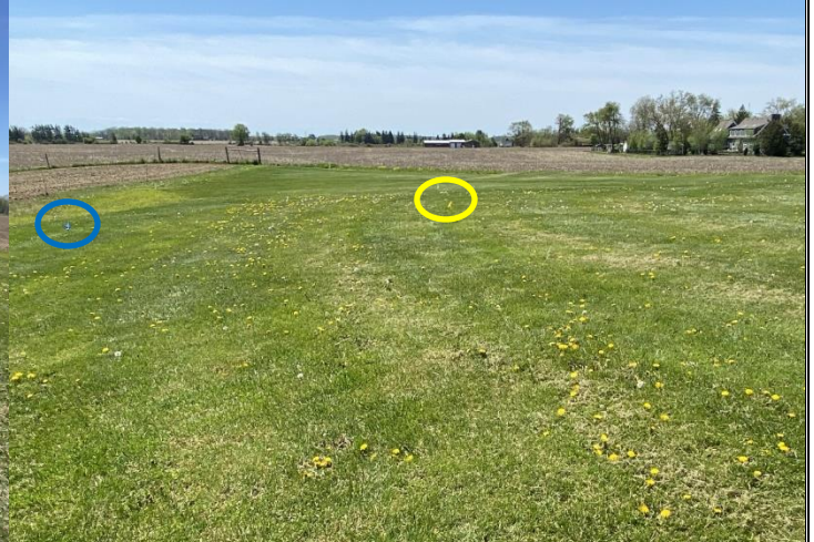
8. End of leaching field distribution lines – yellow flag represents end of lines (11.5m from property) blue flag is the 5m required setback
