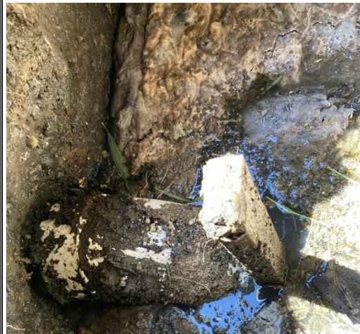
5. 90 degree elbow baffle installed 4 years prior – air locking system causing high levels
