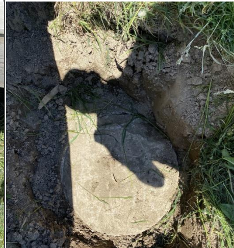
2. Septic tank discharge lid
