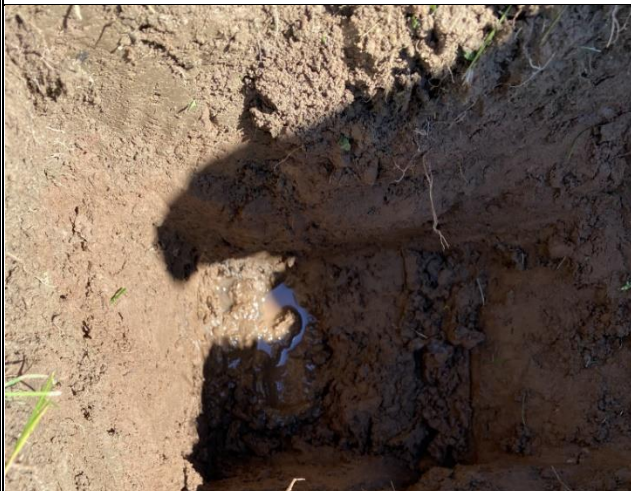
11. Leaching field saturated – water above distribution pipes
