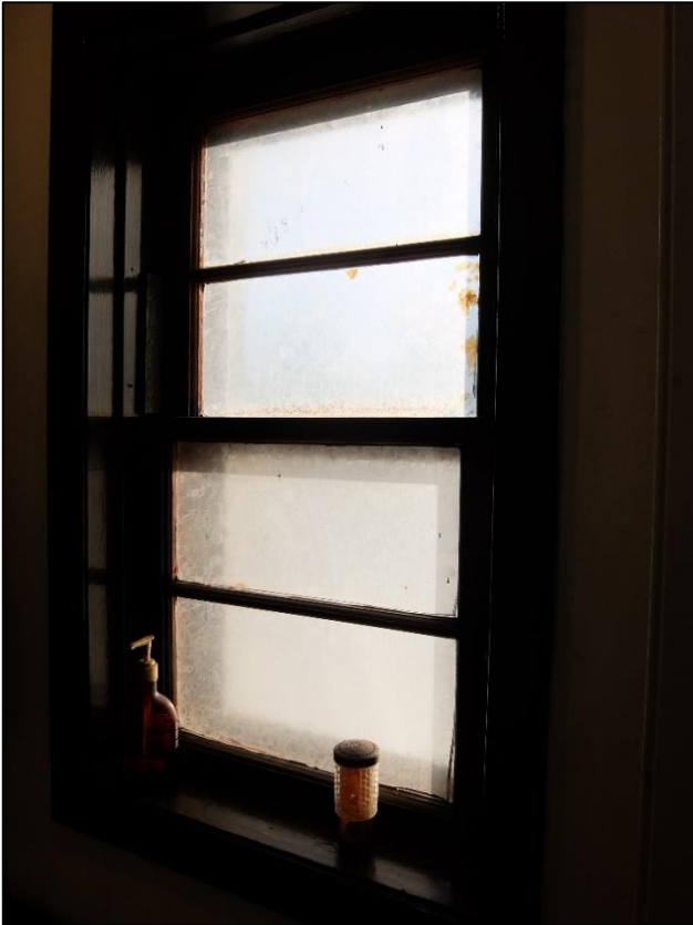
Image 15: Only remaining hung wood window found in the first-floor bathroom, with two-over-two horizontal wood muntins and modern replacement glass and aluminum exterior storms, December 2021 (City of Hamilton)
