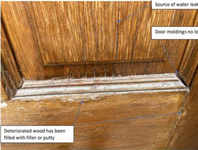
Wood door panels are split. Source of water leaks.
