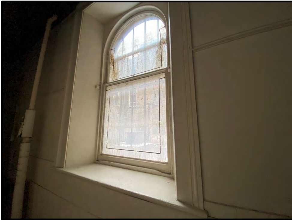
Image 91: First Floor North Addition – Window Opening (Photo taken on December 8, 2021; Facing Southwest)
