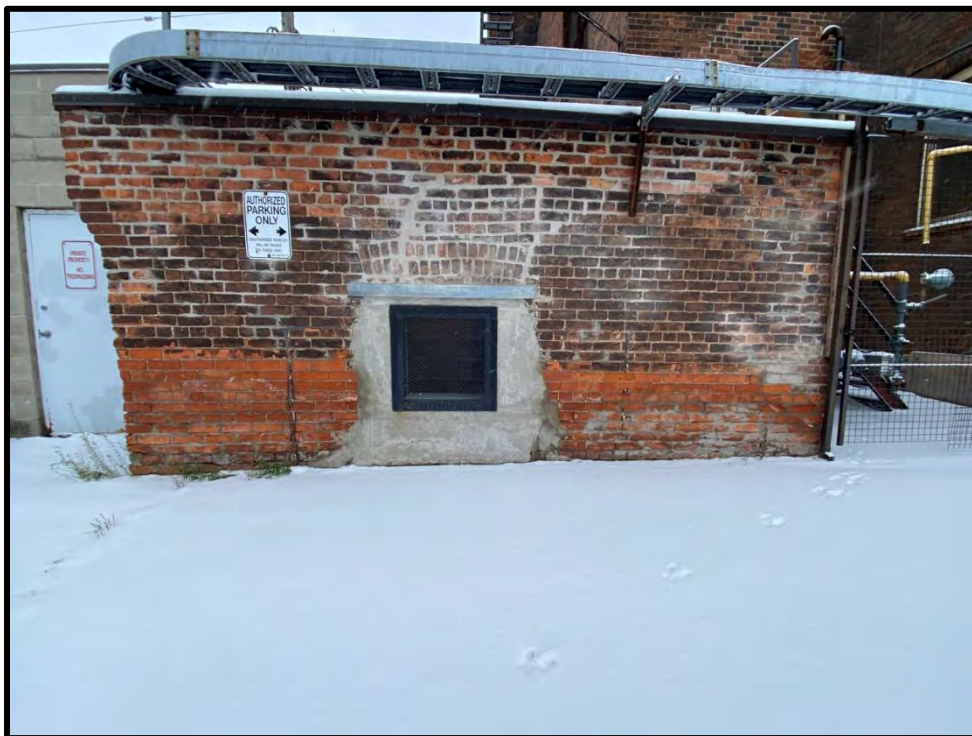
Image 48: Addition at North Part of West Elevation – Detail (Photo taken on December 8, 2021; Facing East)
