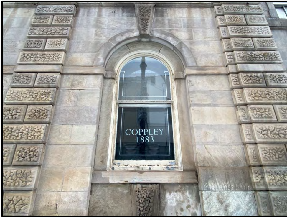
Image 7: First Storey Window Opening and Vermiculated Ashlar Pilasters – Detail (Photo taken on December 8, 2021; Facing North)
