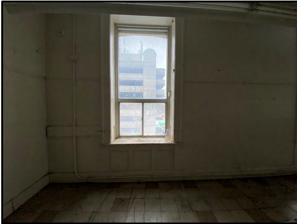
Image 107: Second Floor Stone Building – Window Opening and Wainscoting (Photo taken on December 8, 2021; Facing East)
