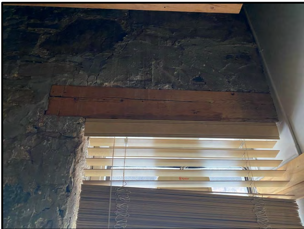
Image 74: First Floor Interior – Wood Sill Detail (Photo taken on December 8, 2021; Facing West)
