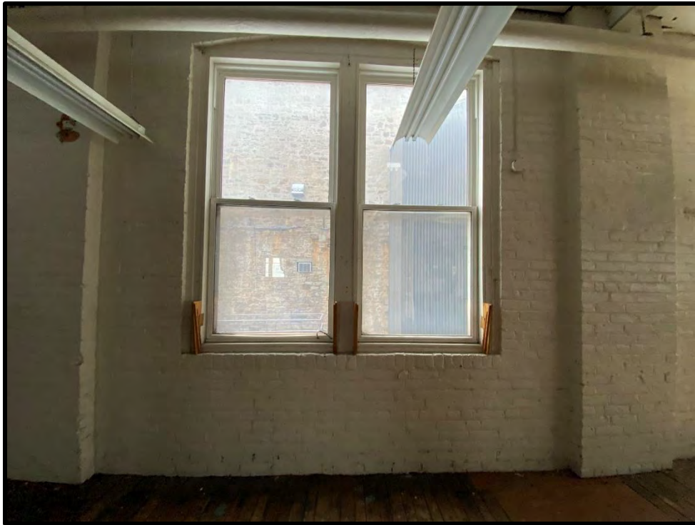
Image 173: Second Floor Brick Building – Window Detail (Photo taken on December 8, 2021; Facing East)
