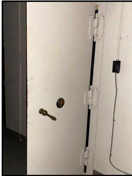
Image 83: First Floor North Addition – Vault Detail (Photo taken on December 8, 2021; Facing Southwest)
