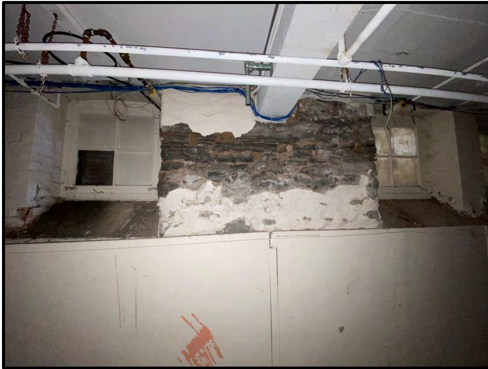
Image 185: Basement Brick Building– Stone and Window Detail (Photo taken on December 8, 2021)
