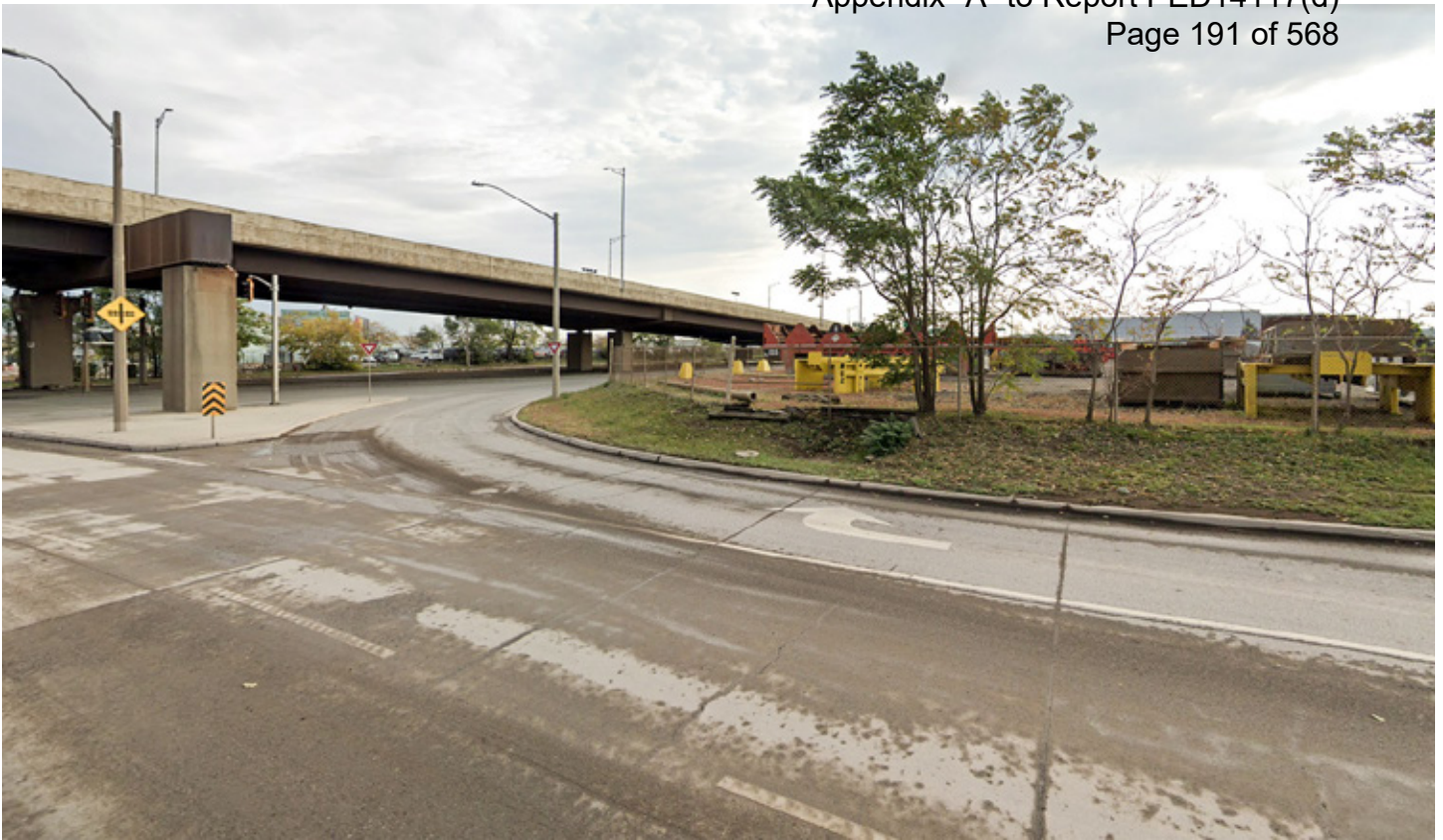
Existing Condition at Kenilworth Ave. N and Burlington St. E. Credit: City of Hamilton
