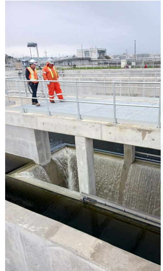
Tertiary Treatment - Woodward WWTP
