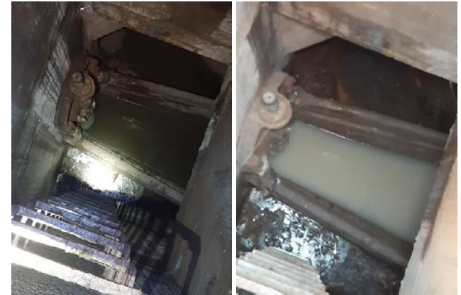
Dunn Ave – suspended trough regulator
