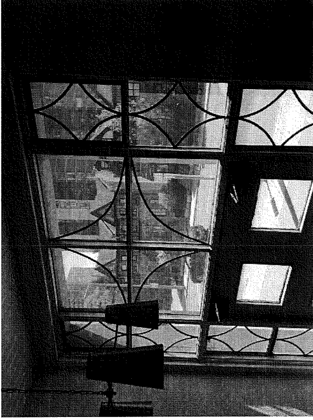
Interior view of 220 Main Street, taken inside the front addition, looking towards Main Street, and the new front entrance assembly. Windows are painted metal units with single pane glazing with lead came.
