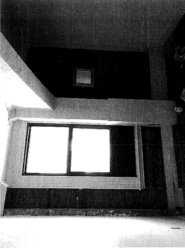
Across: Overall view of the west elevation, seen from Queen Street. The new structure partly obscures the elevation and some ground level openings appear to be later modifications. Some stepped cracking is noted above a second storey window opening, likely as a result of building alterations on the south portion of the structure.
