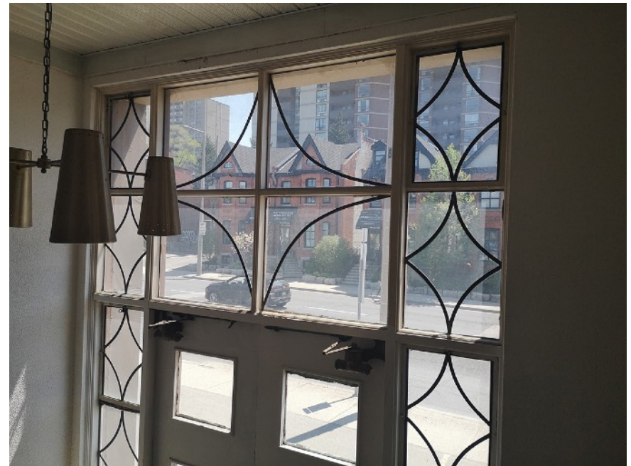
Interior view of 220 Main Street, taken inside the front addition, looking towards Main Street. and the new front entrance assembly. Windows are painted metal units with single pane glazing with lead came.
