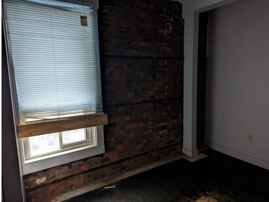
115-117 George Street, Interior Room City of Hamilton, January 20, 2023
