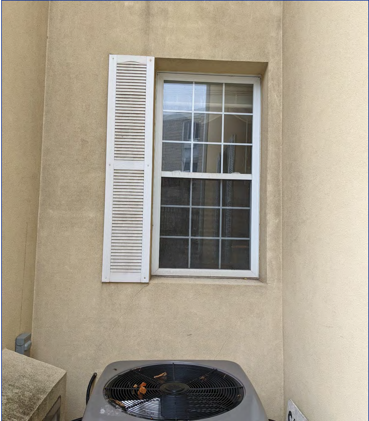
Figure 28: View of the windows in the sunken section of the east elevation
