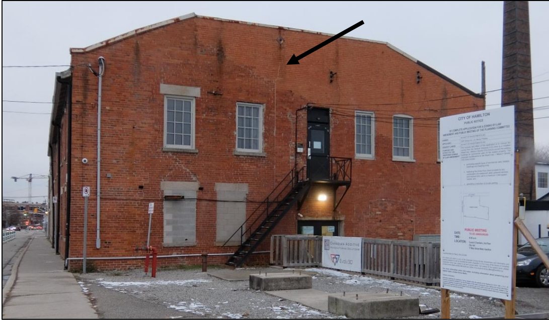
Figure 17: West wall of Building Nos. 2 and 5. Notice the difference in the colour of the brick, marking the former roofline of Building No. 2 (December 2022)
