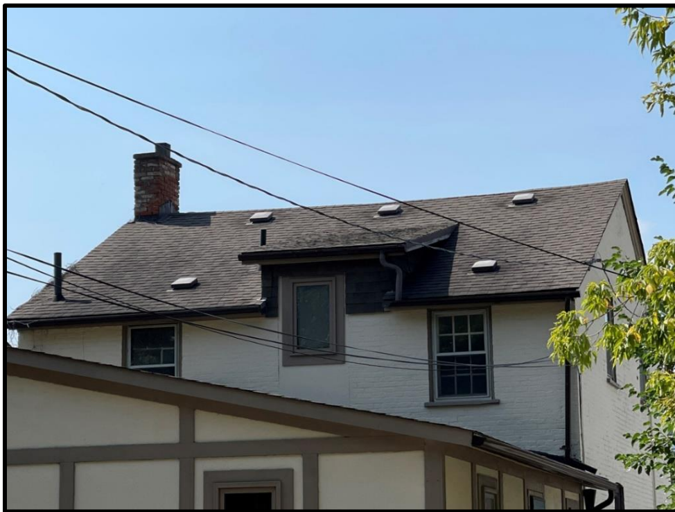
Image 22: North Elevation of Brick Building – Showing Former Door Opening on Dormer at 215 King Street West (Photo taken on August 6, 2021; Facing South)
