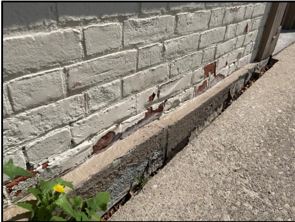
Image 13: 215 King Street West Elevation Brickwork in Flemish Bond Showing Signs of Deterioration (Photo taken on August 6, 2021; Facing North)
