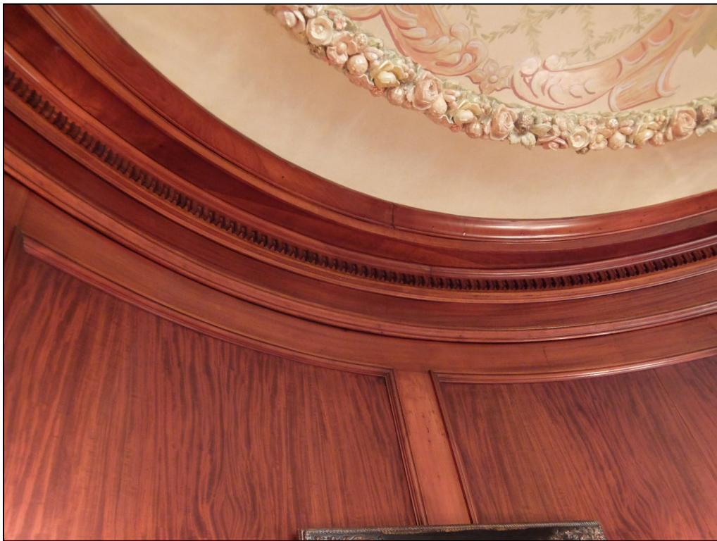
Closeup of the dining room wood carved crown moulding with dentils and ceiling plaster decoration
