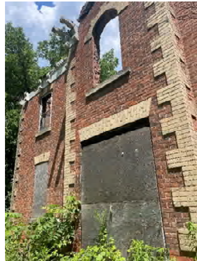
Figure 18 Exterior view of the front of the house showing the boarded front door entry.
