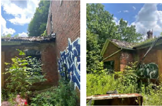
Figure 8 Rear Façade and Garage Graffiti
