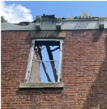
Figure 14 View of one of the remaining window frame on the front façade. These do not appear to be original and are in a damaged state.
