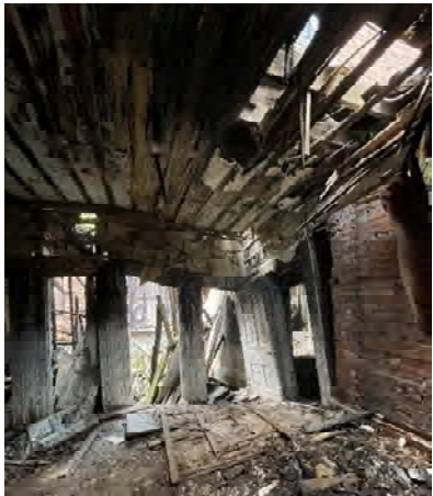
Figure 23 Interior view of the house showing the collapsed second floor. The second floor has collapsed down to the basement in the main portion of the house.
