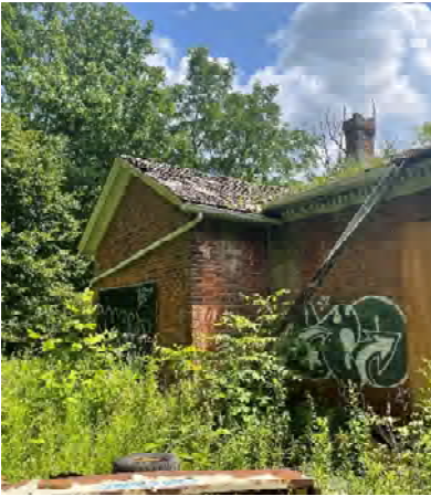
Figure 11 View of remaining damaged soffits to the rear of the house above the garage.
