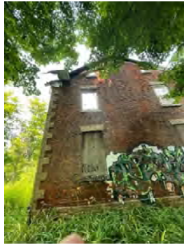
Figure 7 East Façade Graffiti
