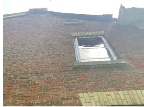
Figure 15 One of the remaining windows was damaged by the fire (West façade second-floor)
