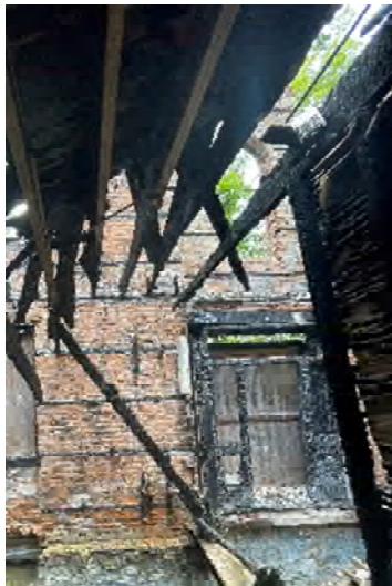
Figure 17 Interior view of the front of the house showing the charred remains of the front door. This is not in a salvageable condition.
