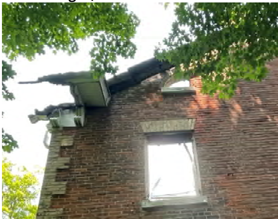
Figure 9 View of the damaged eaves trough and brackets. This is a typical condition of the soffits, fascia and brackets.
