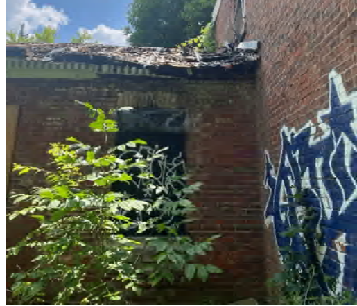
Figure 12 Collapsed roof, rotting soffits and eaves troughs to the rear of the house above the garage
