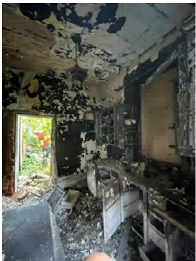
Figure 24 Photo showing existing damage to interior plaster and ceiling moldings.
