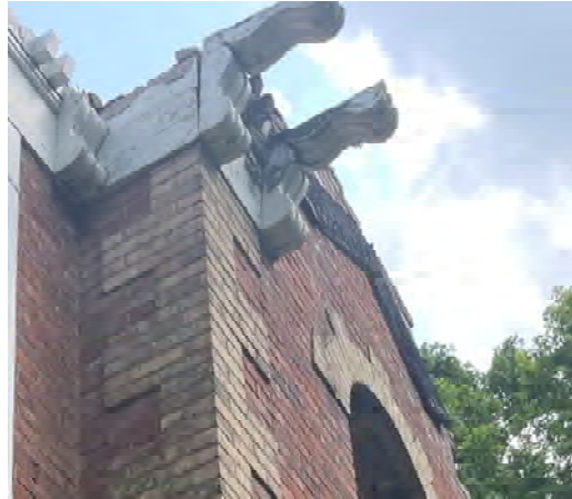
Figure 13 View of damaged brackets at the second level of the front façade.
