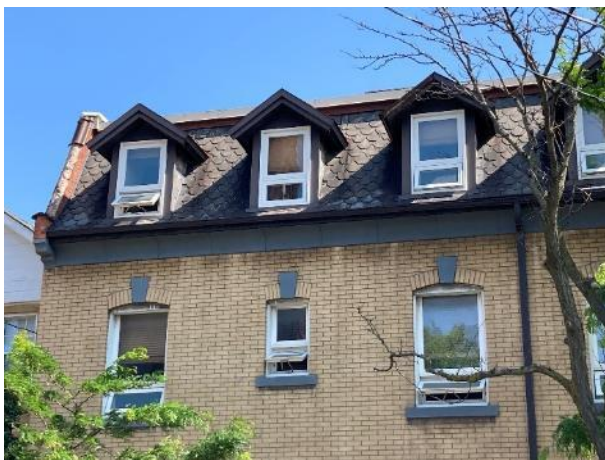
Image 7: Detail of concave mansard roof with scalloped slate tiles and dormer windows
