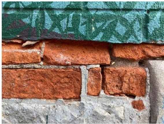
Image 6: Detail of exposed red brick foundation and brick veneer on east side of south elevation
