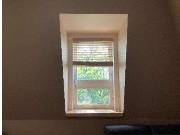
Image 82: Recessed window in south wall of third floor common room, looking south
