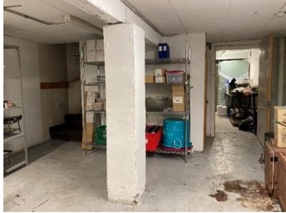
Image 88: View of concrete column and concrete board formed ceiling in basement of addition
