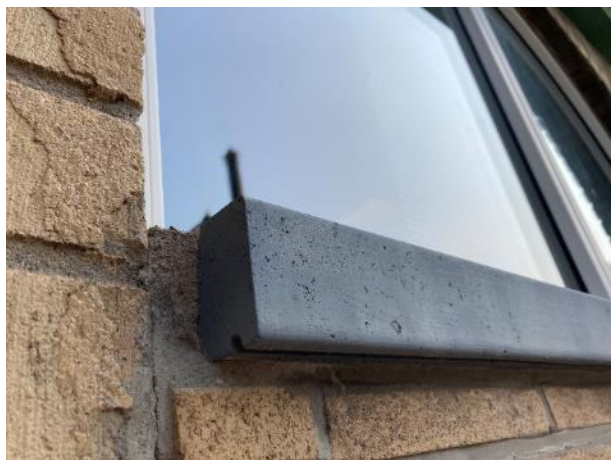
Image 14: Detail of smooth concrete finish of window sill on ground level of south elevation
