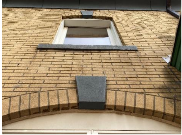
Image 16: Detail of keystone on lower and upper storey window on south elevation
