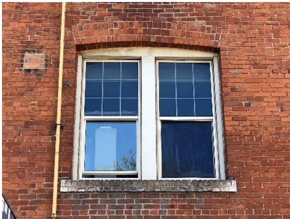
Image 118: Detail of segmentally arched window in west elevation with brick lintel and sill
