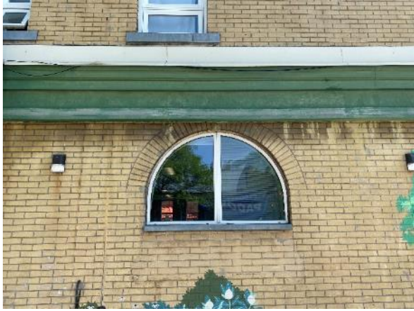
Image 21: Detail of arched window opening and cornice on east side of south elevation
