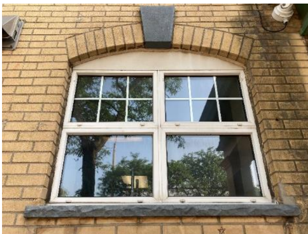
Image 13: Detail of faux etched concrete window sill on main level of south elevation
