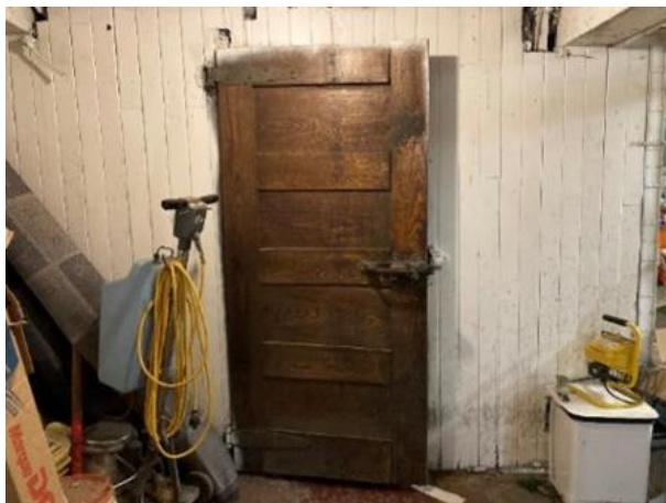
Image 97: Wood panel door leading to walk-in cold storage
