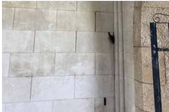
Fig. 38. Missing piece of marble veneer.
