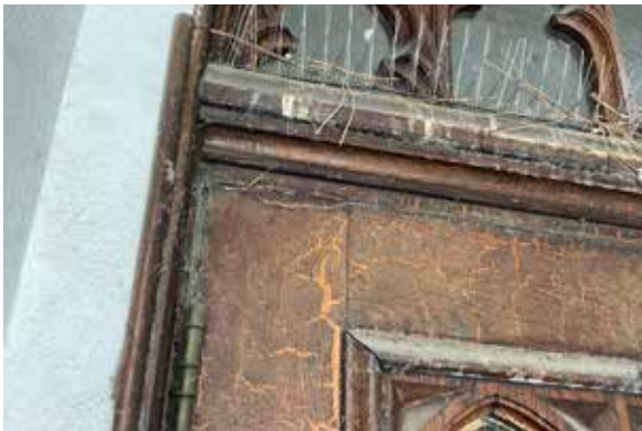
Fig. 83. Broken section of moulding below transom.
