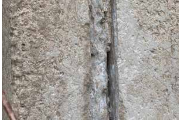
Fig. 27. Evidence of patch repair damage to stone.
