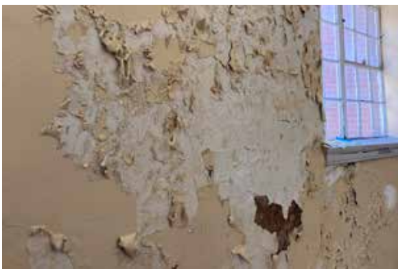
Fig. 104. Moisture damage to plaster and paint.
