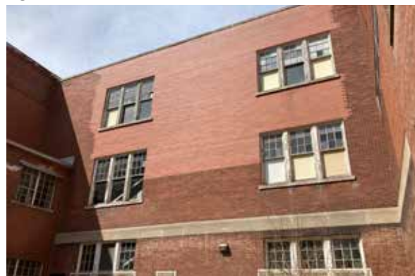
Fig. 45. Unsympathetic brick replacement.
