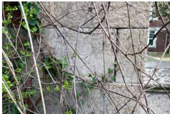
Fig. 29. Washed out joints are visible behind growth.
