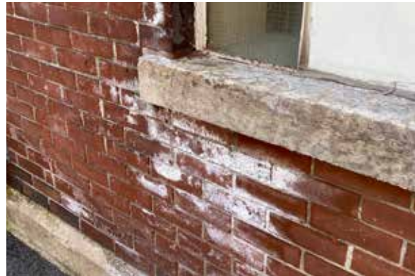
Fig. 48. Severe efflorescence and some spalling.
