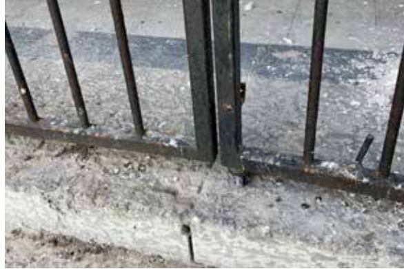
Fig. 26. Damage and staining to steps.
