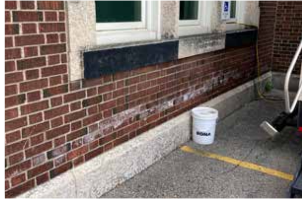
Fig. 18. Example of overpainting on exterior sills.
