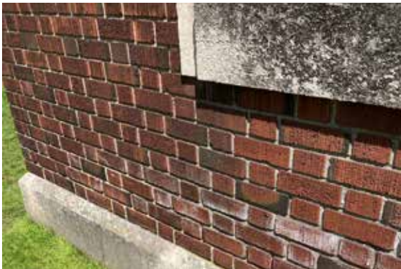
Fig. 3. Example of efflorescence towards base of exterior.
