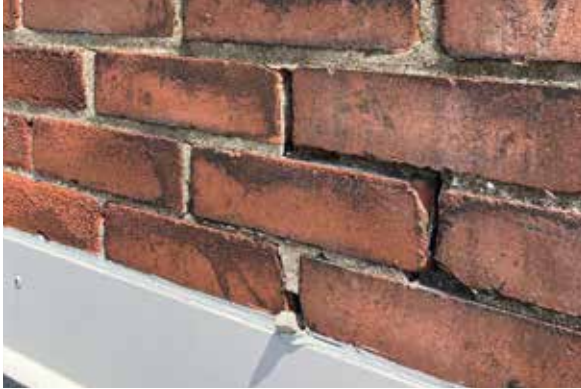
Fig. 71. Significant loss of mortar joints.
