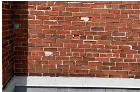
Fig. 67. Evidence of spalled brick and Incompatible repairs.
