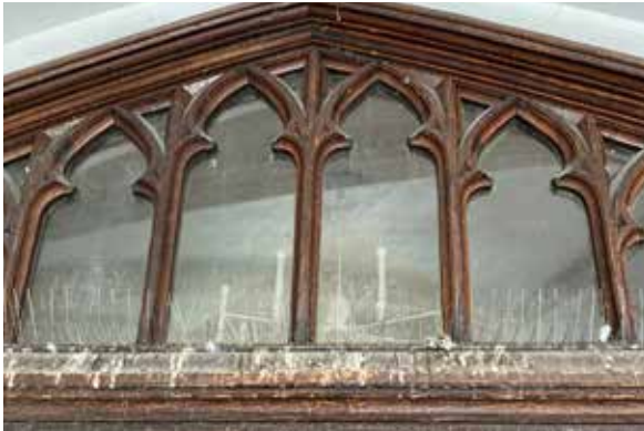
Fig. 82. Bird droppings on otherwise intact transom.
