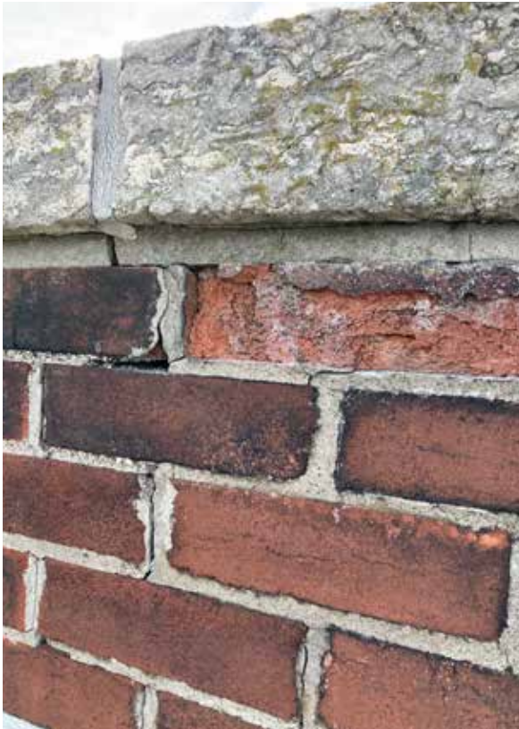
Fig. 72. Mortar cracking between bricks.
