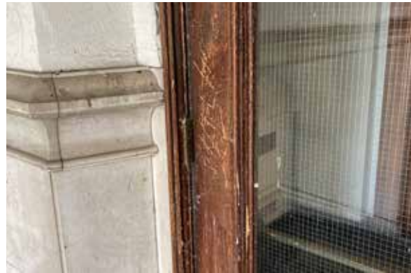
Fig. 78. Surface scratching of northern entrance door.
