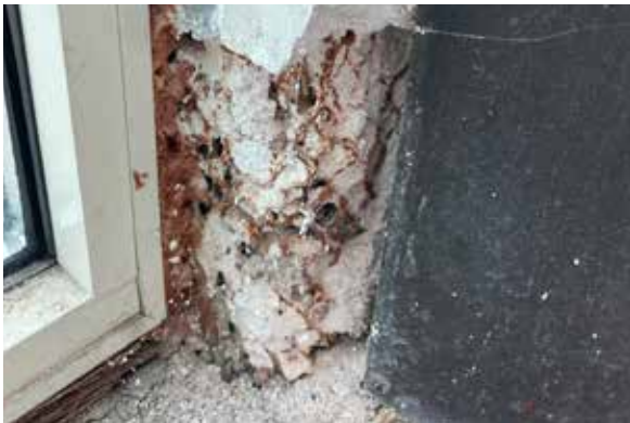
Fig. 108. Failed concrete sill.
