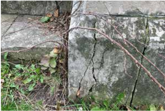
Fig. 23. Large cracks at base of pilasters.
