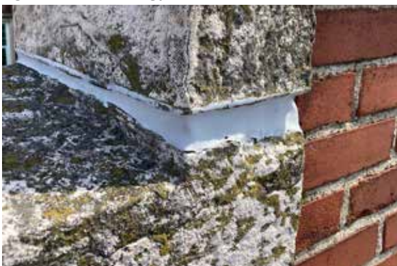
Fig. 59. Pitting, staining and organic growth on parapet.
