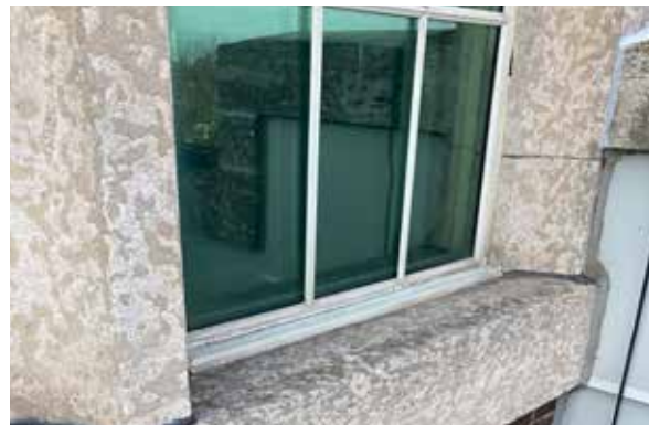
Fig. 33. Washed out joints are visible behind growth.
