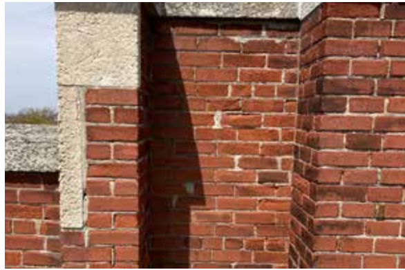
Fig. 75. Incompatible brick replacement (left).
