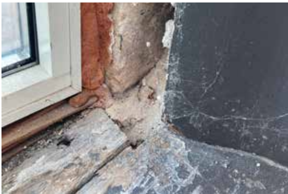
Fig. 109. Failed concrete sill.
