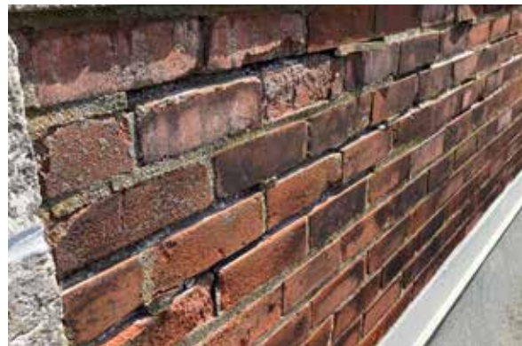
Fig. 69. Spalled brick and loss of mortar joints.
