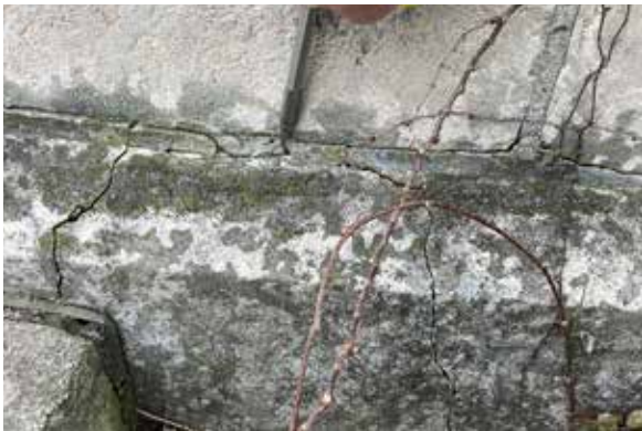
Fig. 24. Large cracks at base of pilasters.
