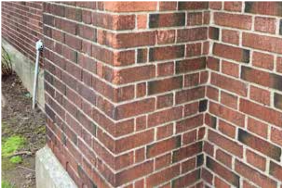
Fig. 2. Example of minimal spalling.
