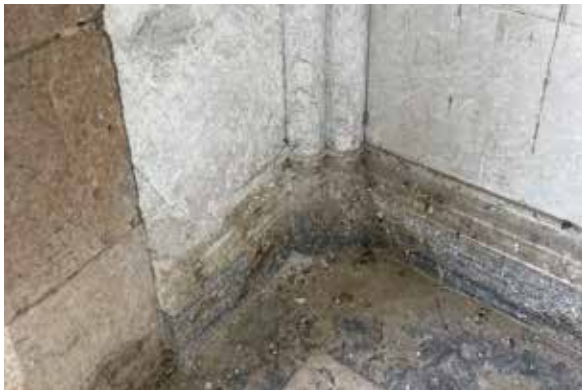
Fig. 36. Soiling at base and floor.
