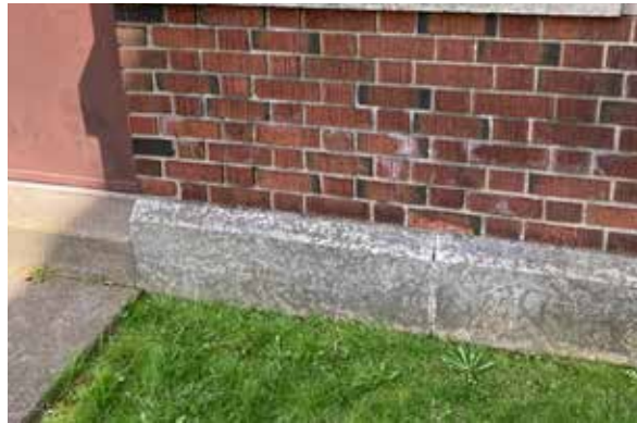
Fig. 6. Example of efflorescence towards base of exterior.
