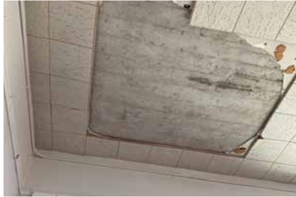
Fig. 111. Missing ceiling tiles and exposed roof deck.
