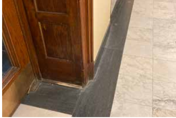
Fig. 97. Main lobby surface wear.
