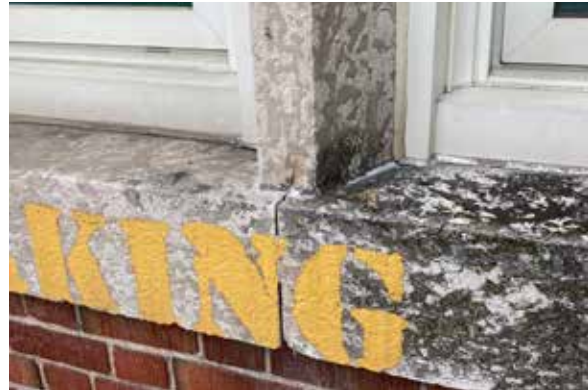
Fig. 20. Example of overpainting on exterior sills.
