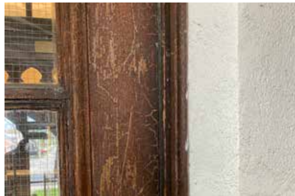
Fig. 79. Surface scratching of northern entrance door.
