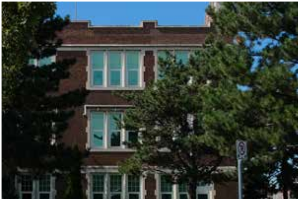
Fig. 11. Evidence of repointing in the lighter areas of brick.
