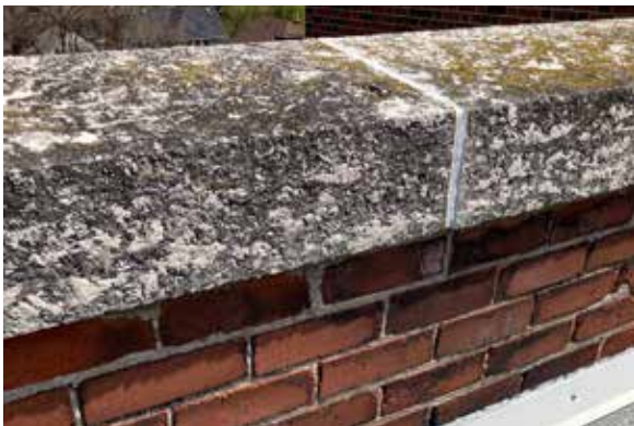
Fig. 65. Area of stone degradation.
