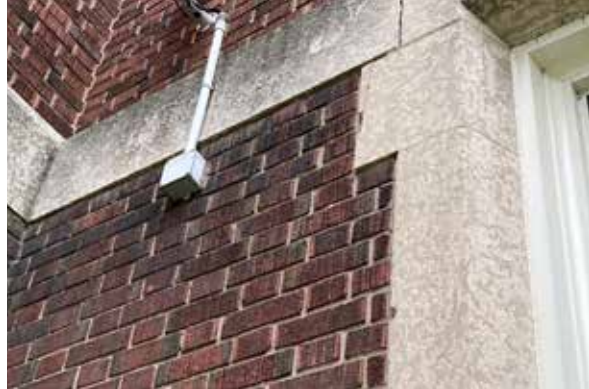
Fig. 13. Areas of minor stone chipping surrounding window.
