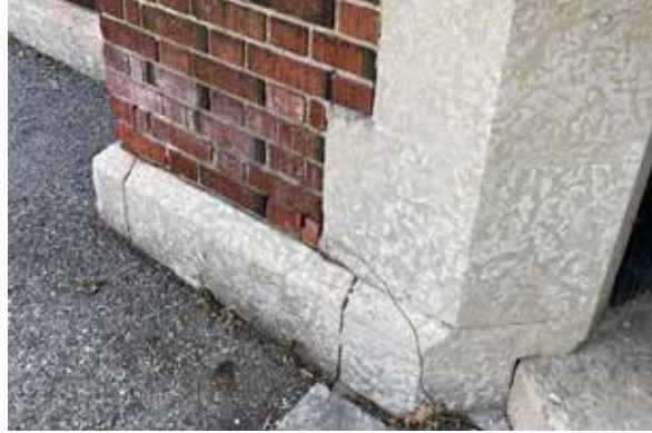
Fig. 5. Example of efflorescence towards base of exterior.
