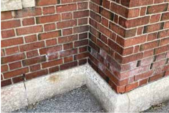
Fig. 1. Example of minimal spalling and efflorescence.
