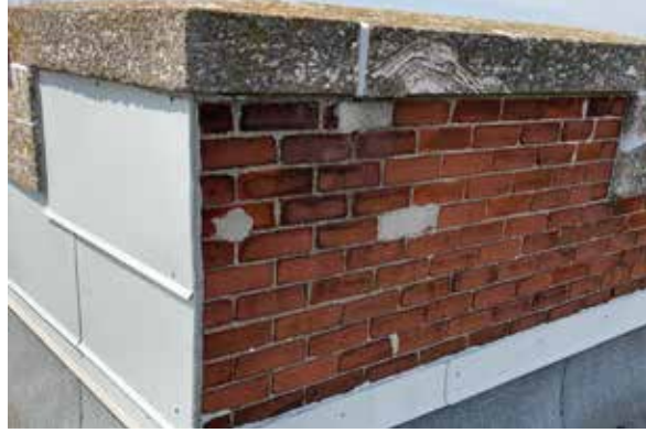
Fig. 73. Incompatible spall repair.
