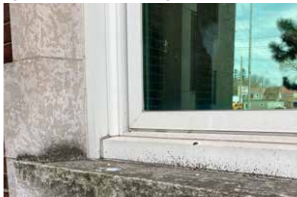
Fig. 16. Significant stone staining and organic growth.
