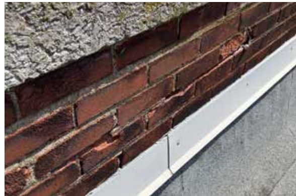
Fig. 68. Chips and spalled brick.
