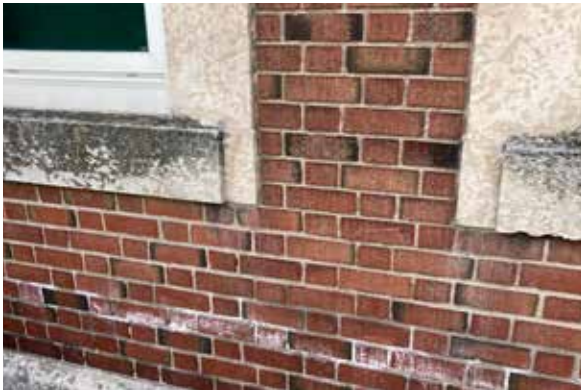
Fig. 4. Example of efflorescence towards base of exterior.
