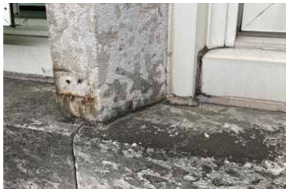
Fig. 15. Example of stone staining, holes and rust.
