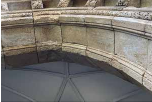
Fig. 22. Moderate pitting and loss of detail in stone arch.
