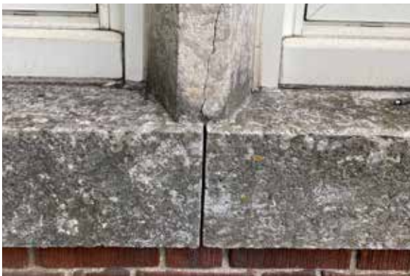
Fig. 12. Example of stone cracking.
