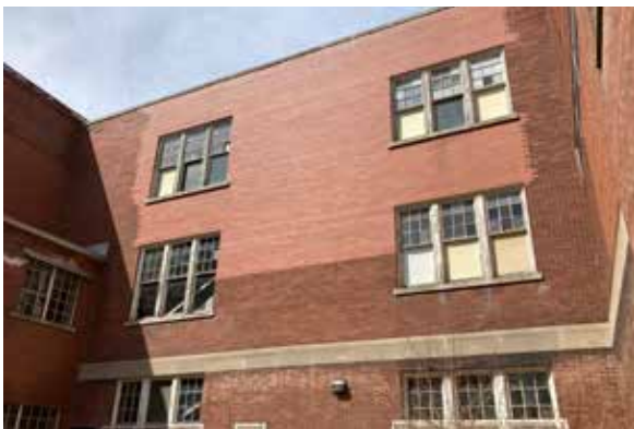
Fig. 53. Unsympathetic window replacements.
