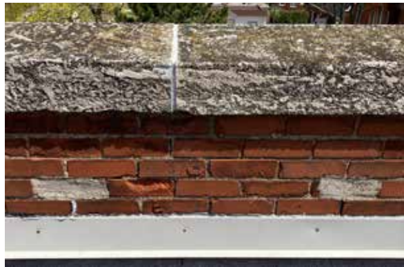
Fig. 76. Incompatible brick replacements.
