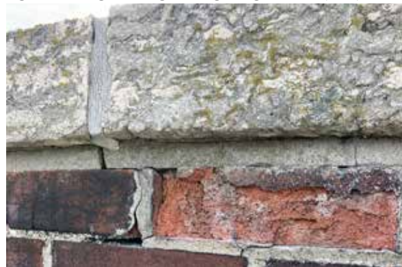
Fig. 61. Failed mortar joint.
