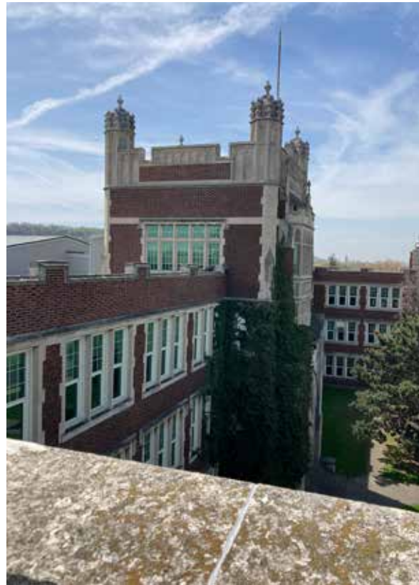
Fig. 31. Evidence of patch repair damage to stone.
