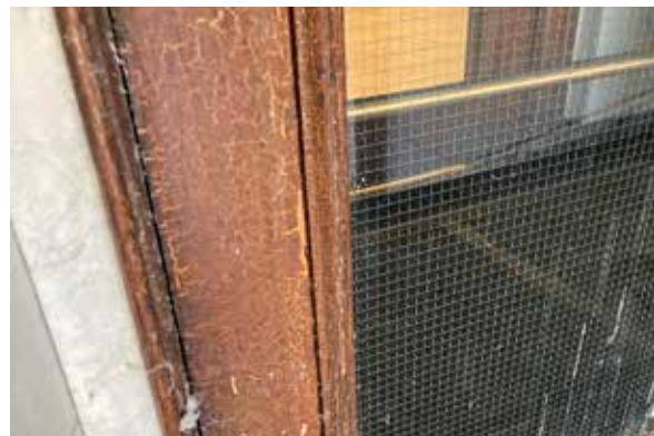
Fig. 80. Crazing of wood coating.
