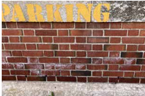
Fig. 7. Example of efflorescence towards base of exterior.
