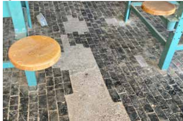
Fig. 116. Block flooring concrete patches.
