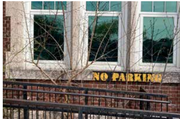
Fig. 19. Example of overpainting on exterior sills.
