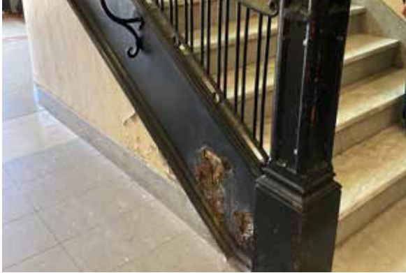
Fig. 106. Corrosion at base of west stair.
