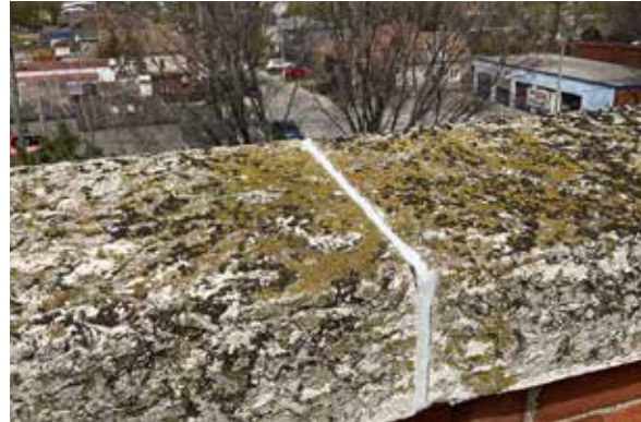
Fig. 60. Pitting, staining and organic growth on parapet.
