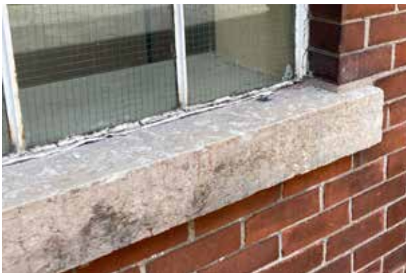
Fig. 58. Failed caulking joints at window sills.
