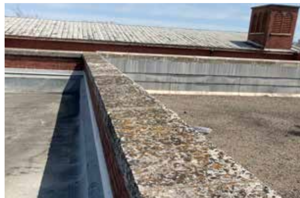
Fig. 63. Pitting, staining and organic growth on parapet.
