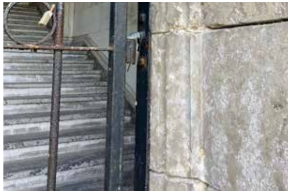
Fig. 14. Example of stone cracking.
