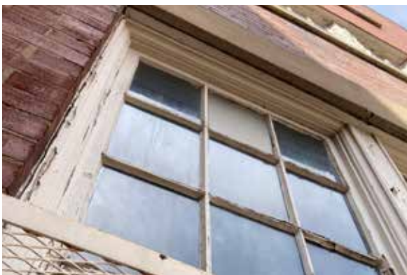
Fig. 54. Large cracks at base of pilasters.
