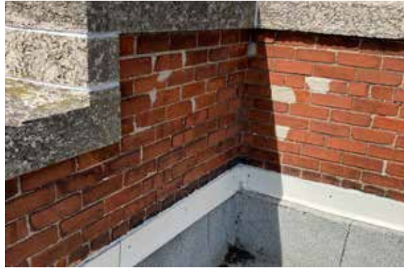
Fig. 74. Incompatible spall repair.
