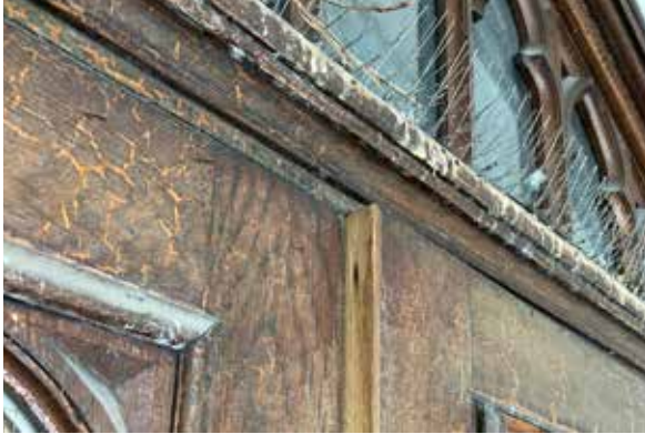
Fig. 81. Cracking of wood coating.
