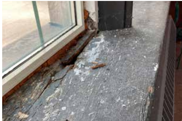
Fig. 112. Deteriorated wooden sills.
