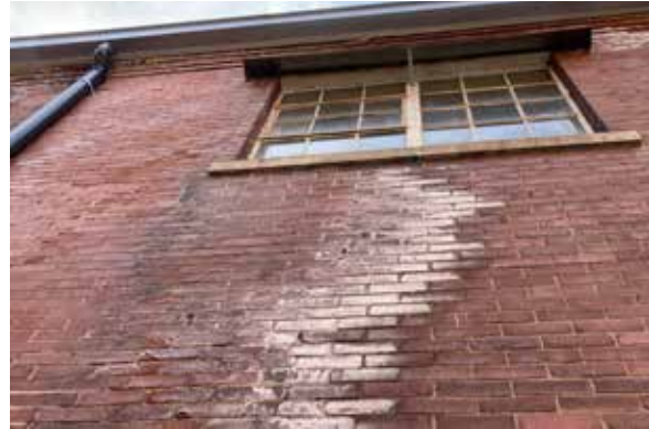
Fig. 47. Severe efflorescence and some spalling.
