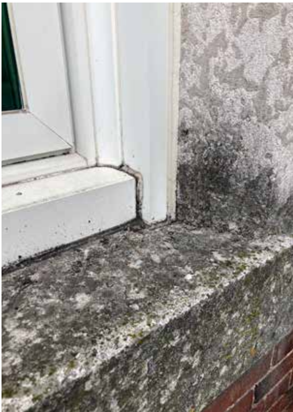
Fig. 17. Significant stone staining and organic growth.
