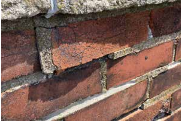
Fig. 70. Brick and mortar failure underneath parapet stone.
