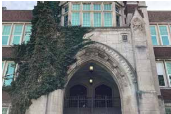
Fig. 28. Growth on the tower impeded proper inspection.
