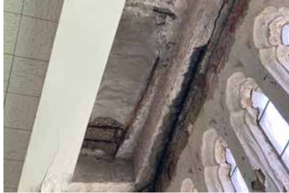
Fig. 110. Deteriorated cement finish.
