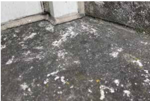
Fig. 40. Debonding between stone and caulking.
