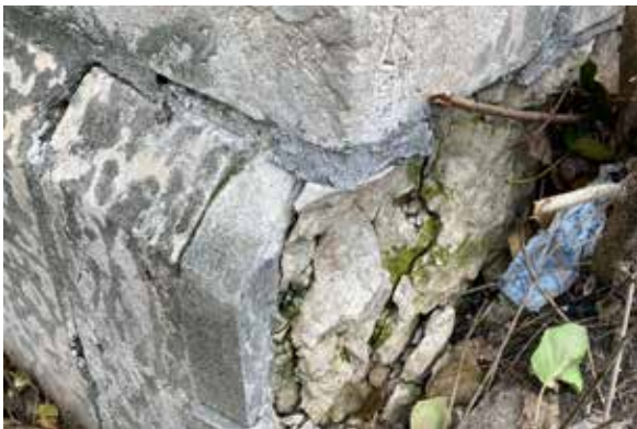
Fig. 25. Large cracks at base of pilasters.
