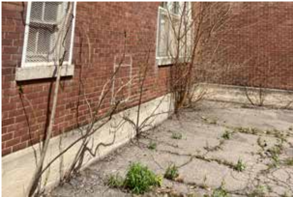
Fig. 52. Vegetal growth at base of north wall.
