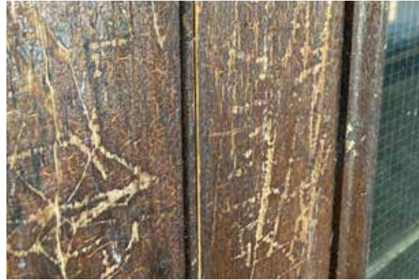
Fig. 77. Surface scratching of northern entrance door.
