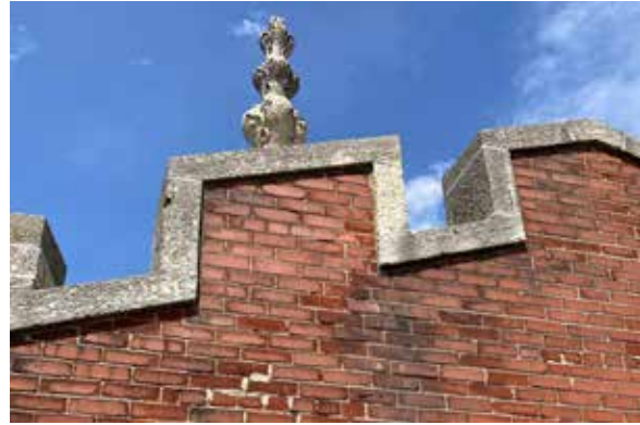
Fig. 66. Area of stone degradation and chipping.
