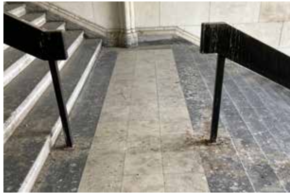
Fig. 37. Soiling at base and floor.
