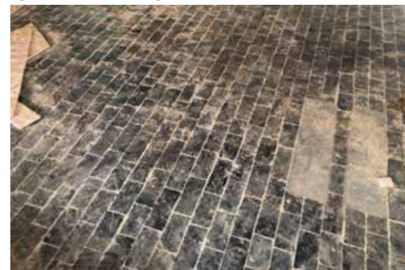
Fig. 117. Block flooring concrete patches.
