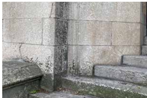
Fig. 21. Eroded stone joints & organic growth.
