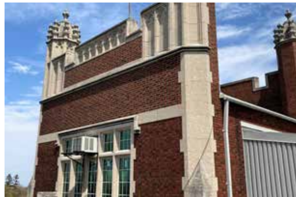
Fig. 32. Growth on the tower impeded proper inspection.
