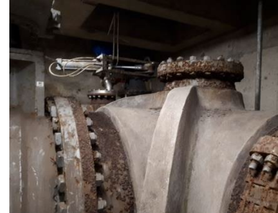
High Lift Pumping Station
