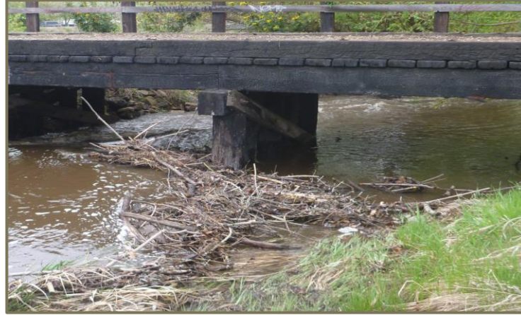
Debris in Creeks
