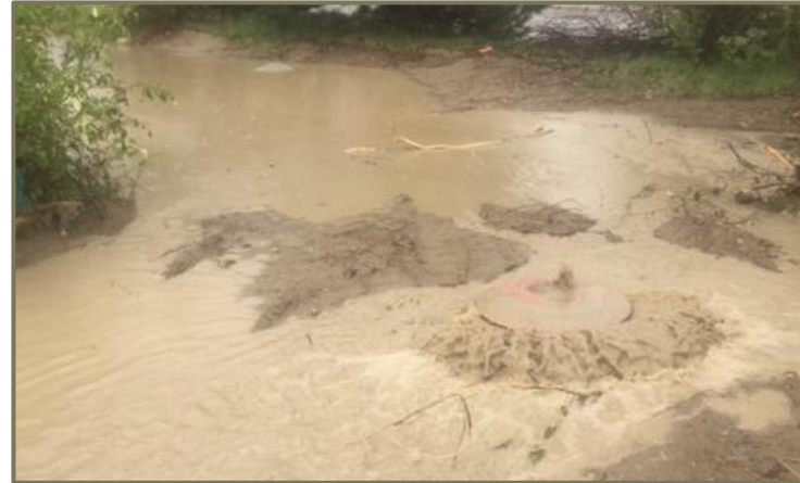
System Surcharge/ Basement Flooding
