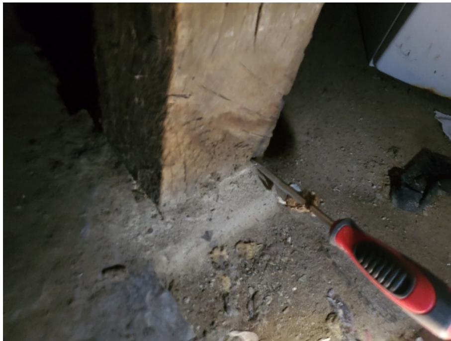
Photo No 08: Rotted Post Base
