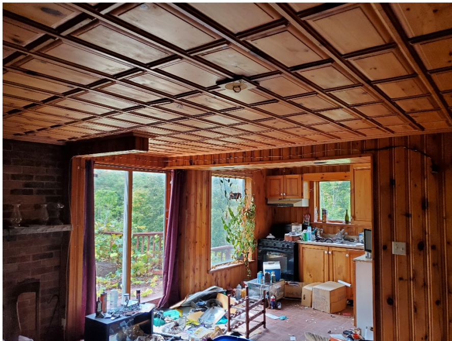
Photo No 02: North Kitchen Wall below Photo No:01
