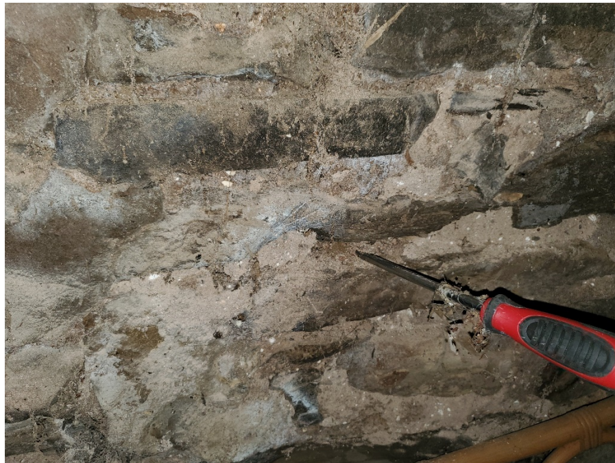
Photo No 10: Spalled Mortar Joint
