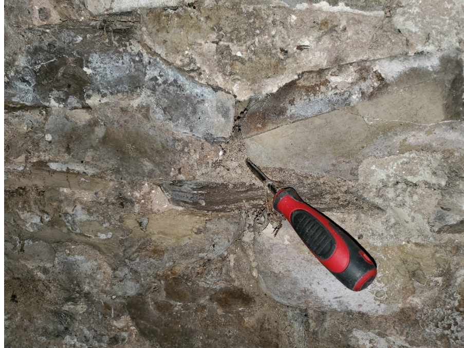
Photo No 11: Spalled Mortar Joint
