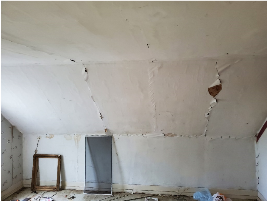
Photo No 01: 2 nd Floor North Wall above Kitchen
