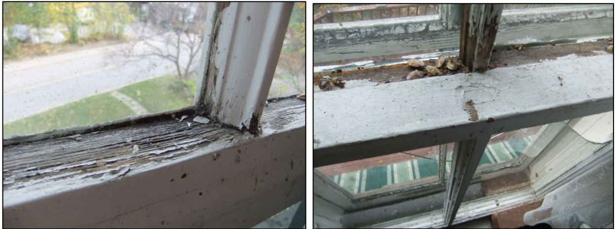
Figure 16: View of deterioration of upper-storey wood windows
