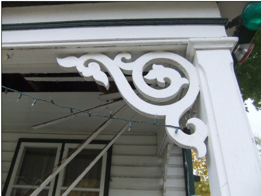
Figure 20: Close-up view of scroll work
