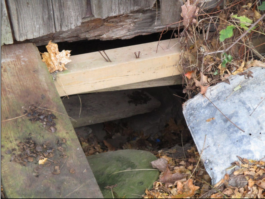
Figure 5: View of damage to shed foundation
