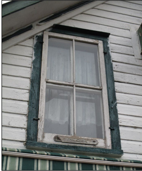
Figure 9: View of deterioration to wooden storm window
