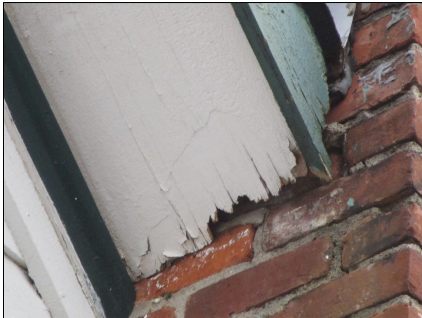
Figure 8: Detail View of damage to eaves
