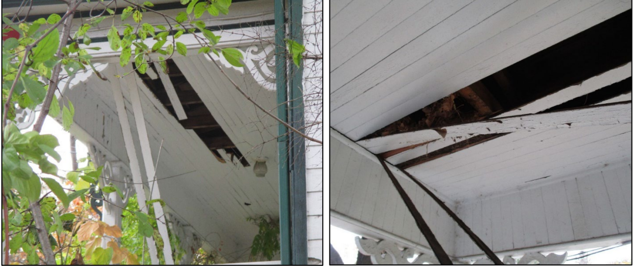
Figure 7: Views of damage to front porch ceiling
