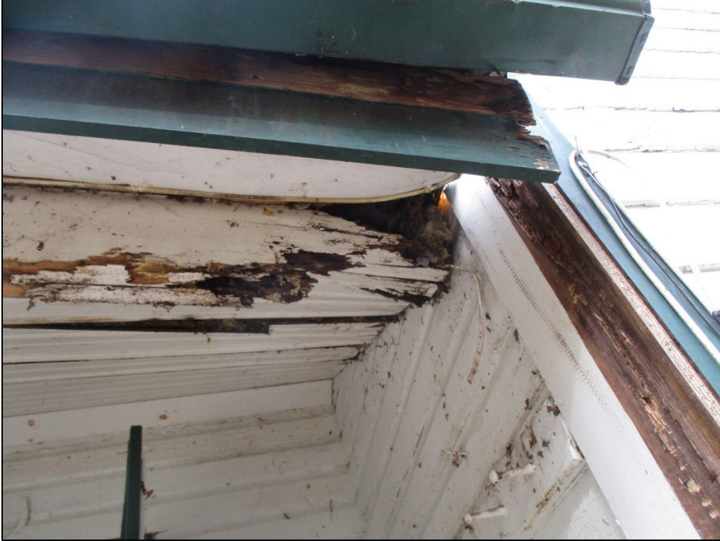
Figure 11: Detail View of damage to side porch
