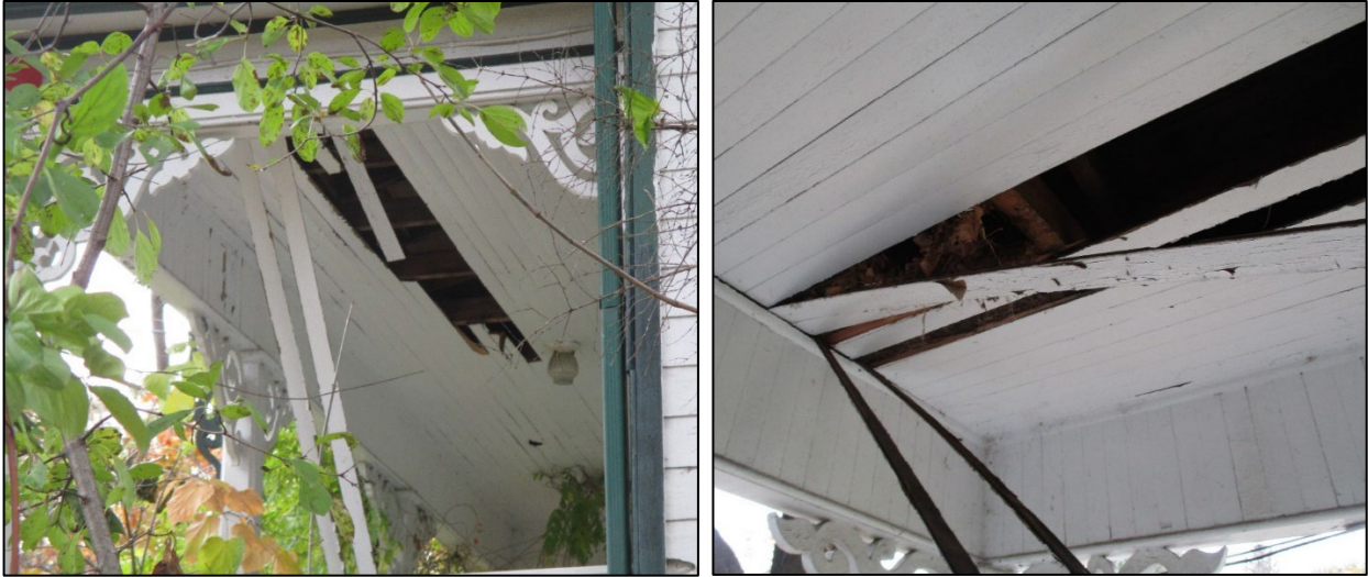
Figure 7: Views of damage to front porch ceiling
