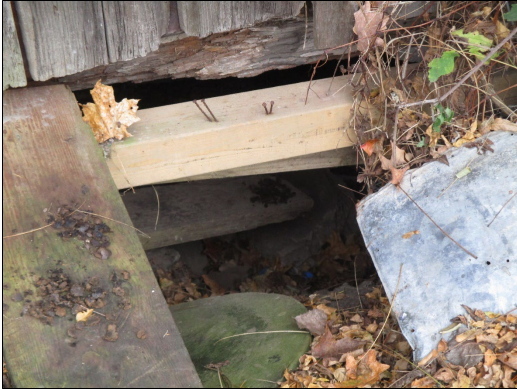
Figure 5: View of damage to shed foundation
