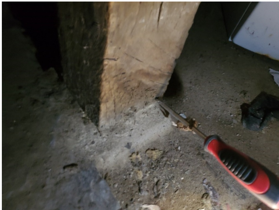
Photo No 08: Rotted Post Base
