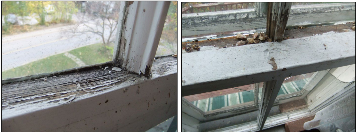
Figure 16: View of deterioration of upper-storey wood windows
