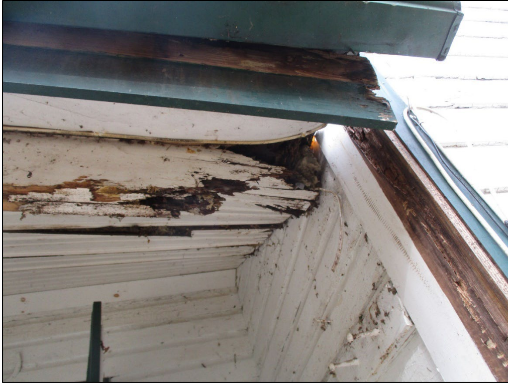
Figure 11: Detail View of damage to side porch
