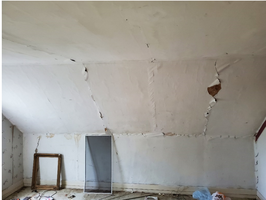
Photo No 01: 2 nd Floor North Wall above Kitchen
