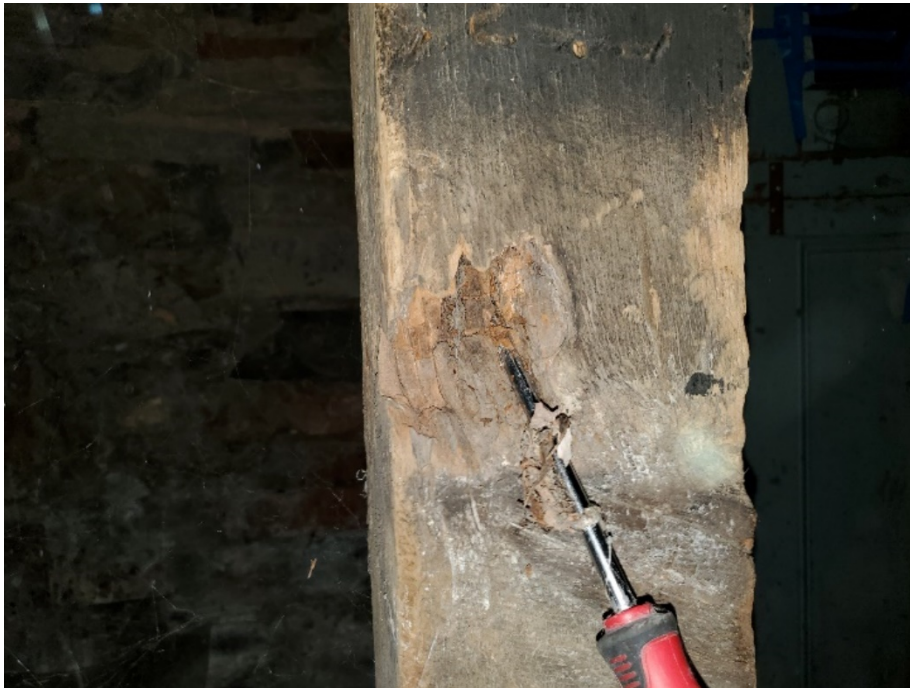
Photo No 09: Rotten Wood Knott
