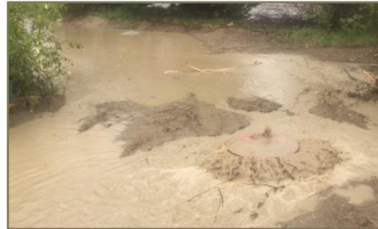
System Surcharge/ Basement Flooding
