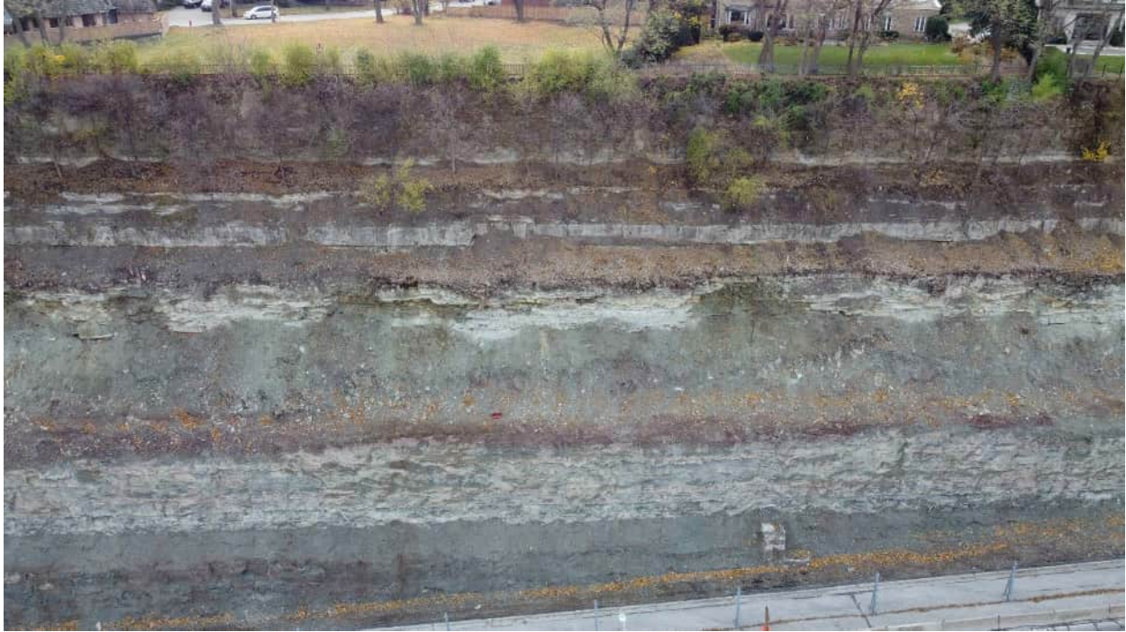
Photo 2. Aerial Imagery of the Escarpment face between the Claremont Access and 14 Belvidere Avenue
