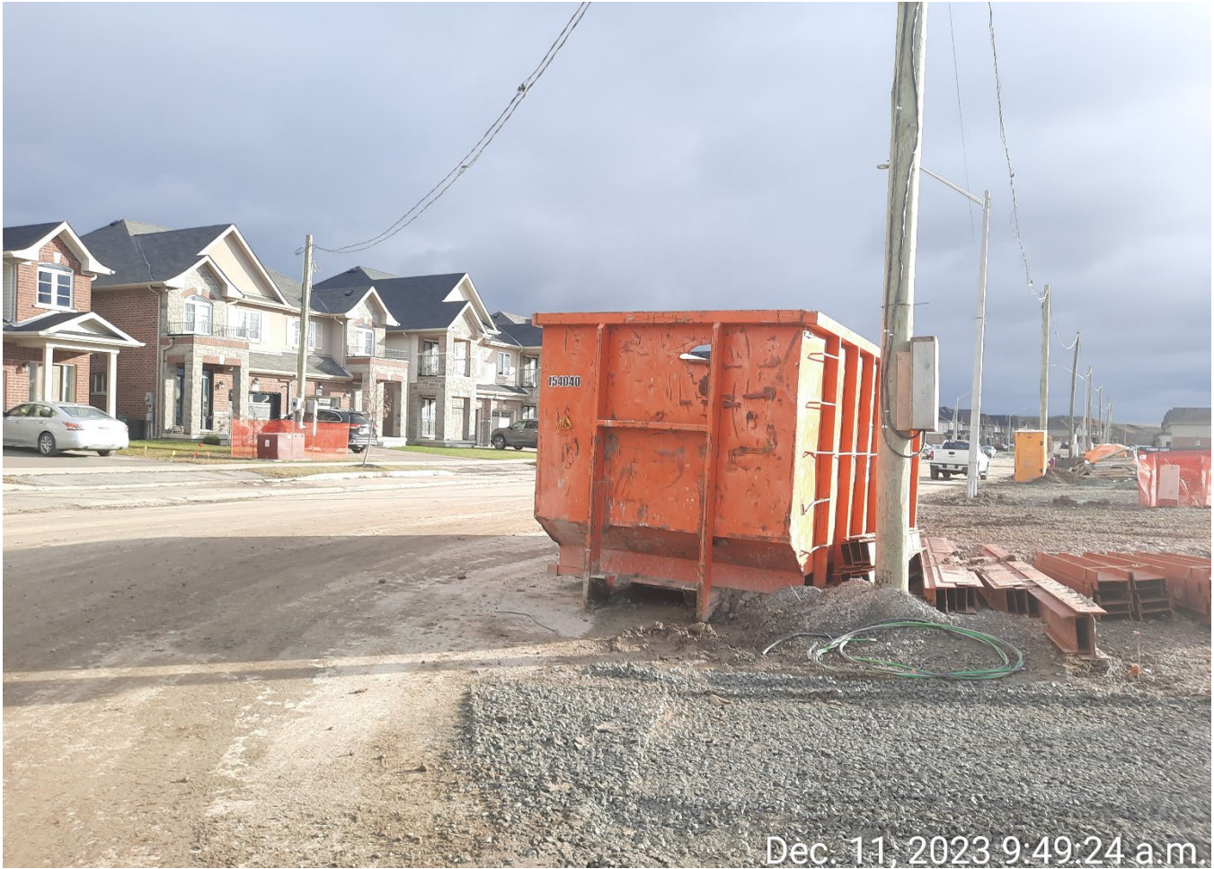
CONTRACTOR'S BIN ON THE ROAD WITHOUT A PERMIT AND CAUSING A SIGHTLINE ISSUE FOR MOTORISTS
