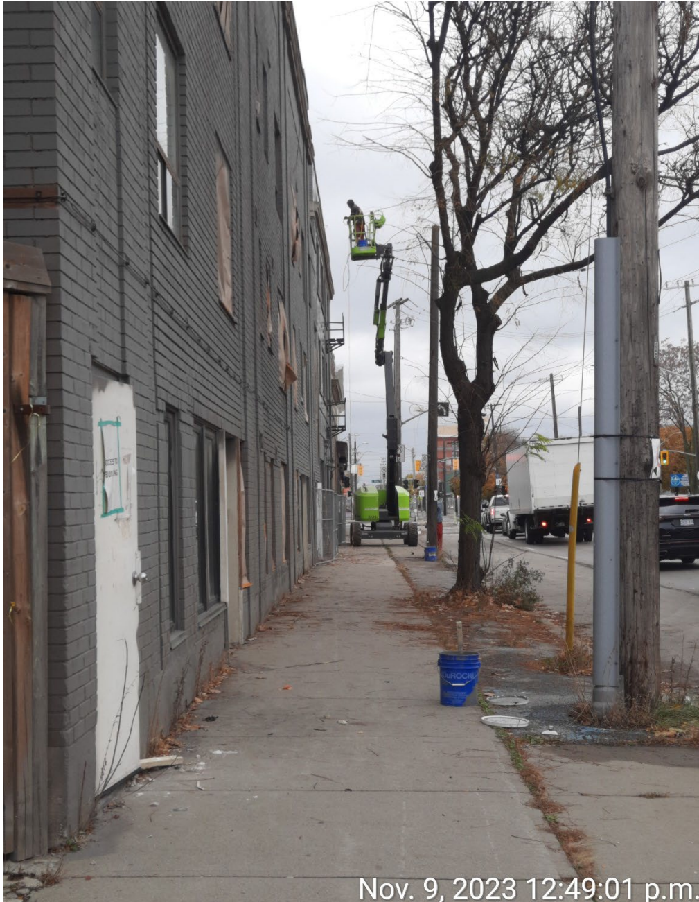
CONTRACTORS LIFT BLOCKING THE SIDEWALK No Occupancy Permit
