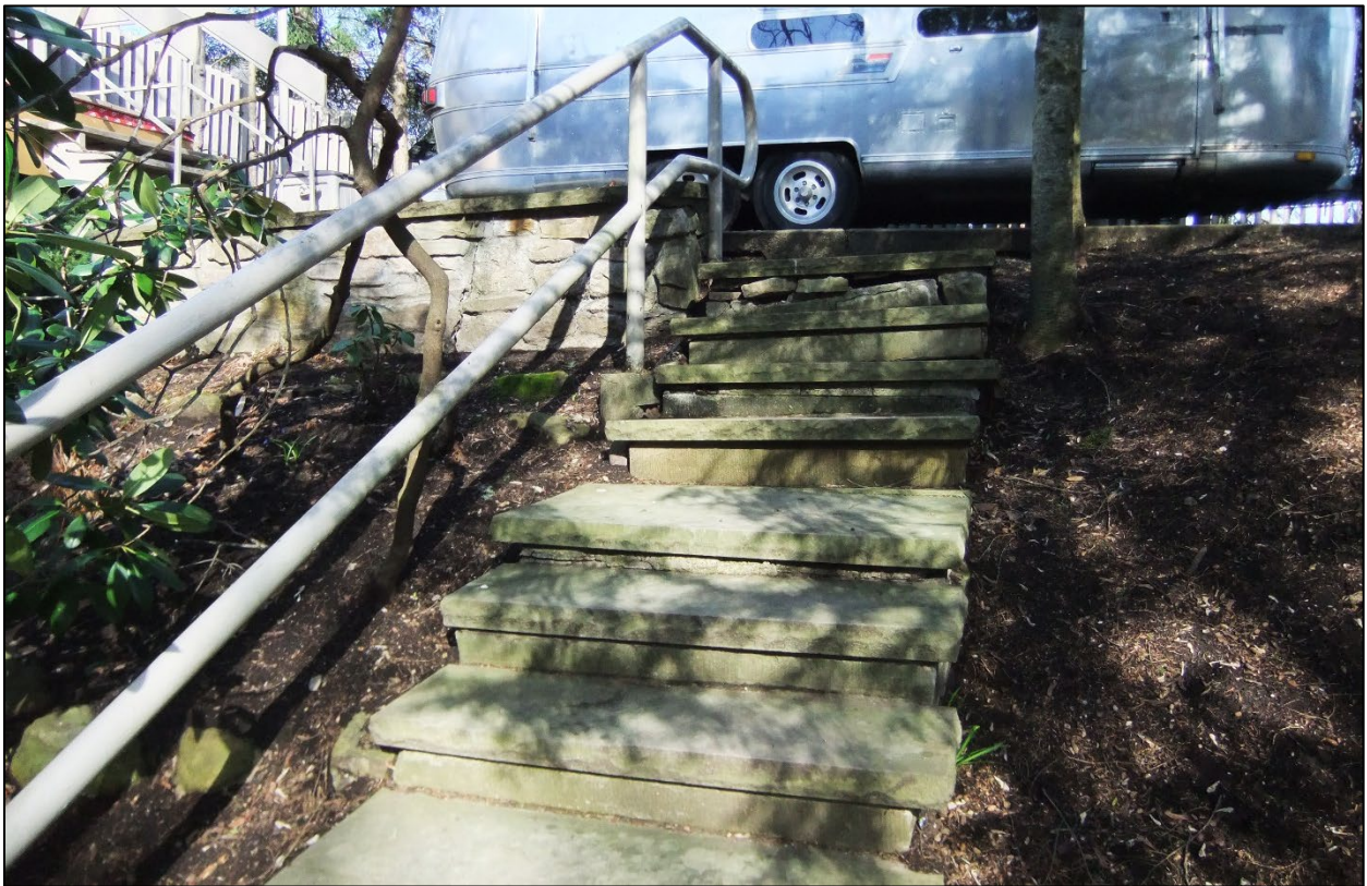
Image 10: Image of cut stone stairs leading down from the upper level entry way and stone planter.
