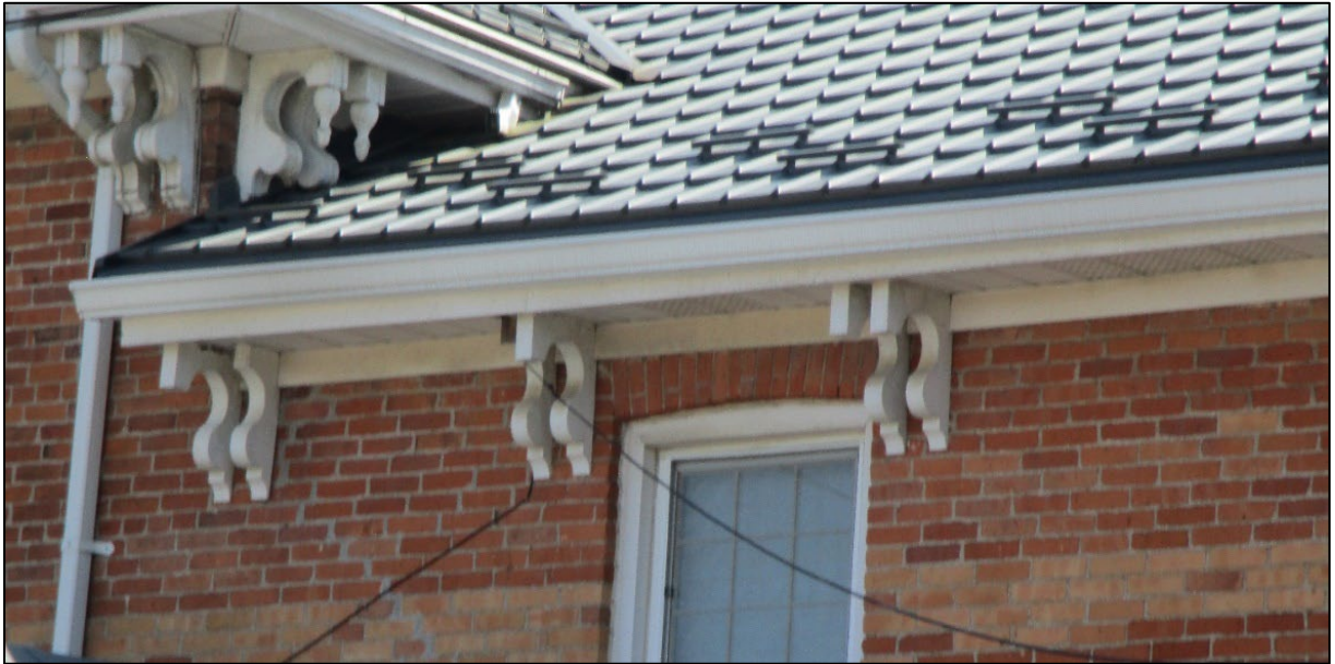
Image 9: Detail of brackets on the north elevation at the intersection of the main building and the rear wing.
