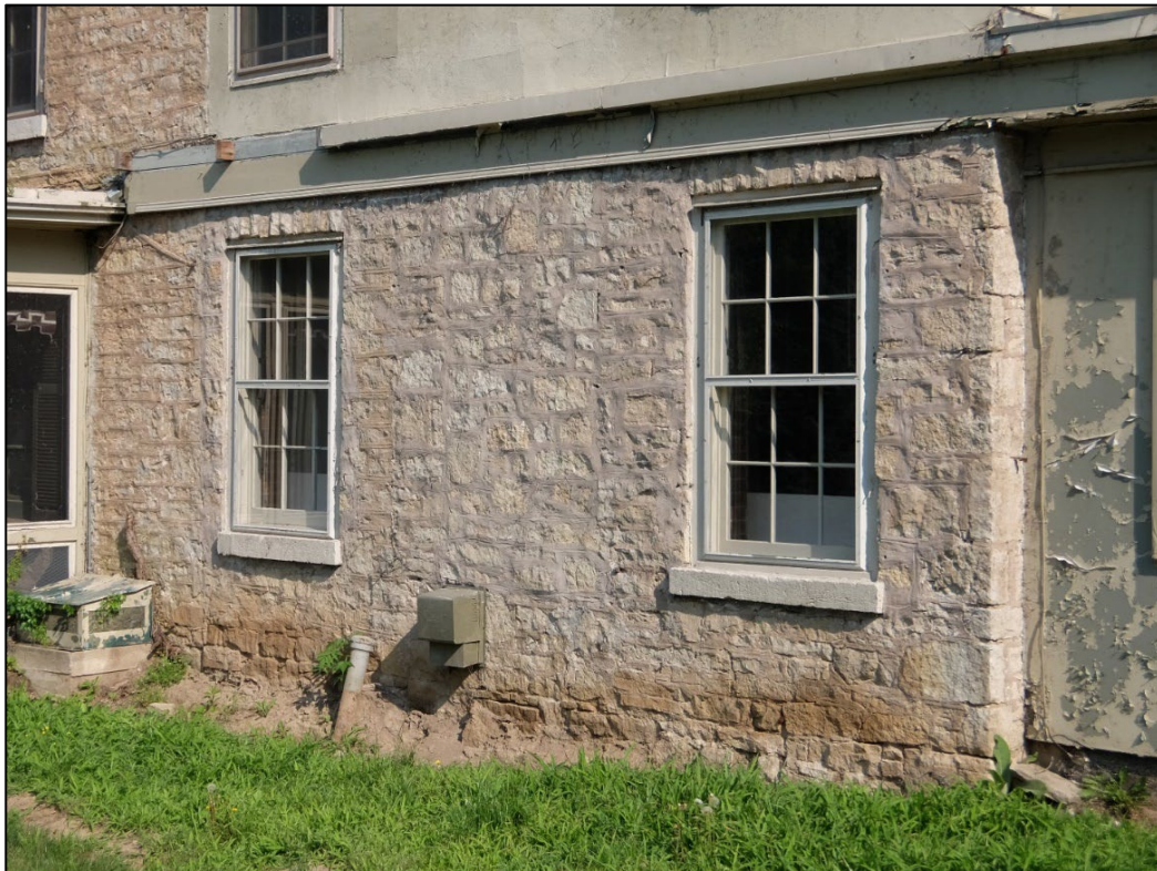
Figure 10: Detail view of the first storey of the circa 1860 eastern side addition.
