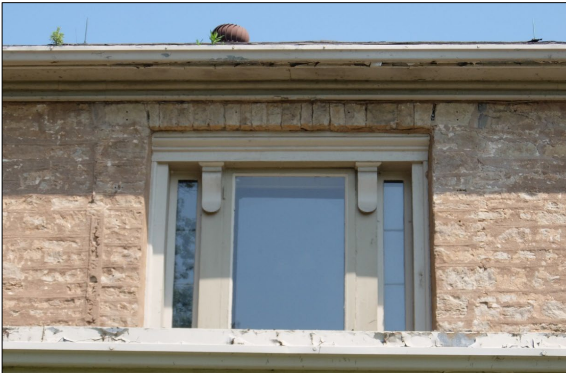
Figure 12: Detail view of Venetian window in the second storey of the south (front) elevation.
